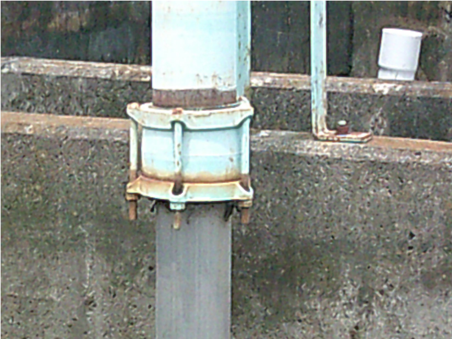
Figure 5: Image of the carbon to stainless steel connection.
