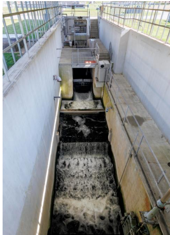
Figure 2- One Channel UV System in use
