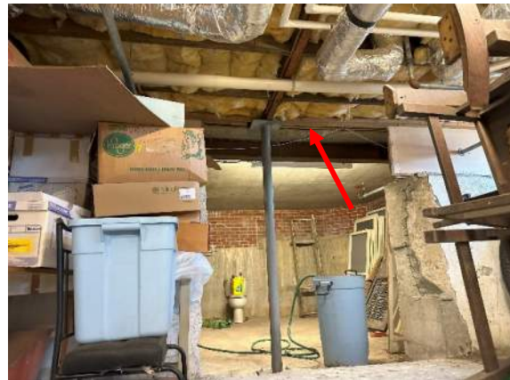
Picture 4 – Example of area of reported water intrusion
