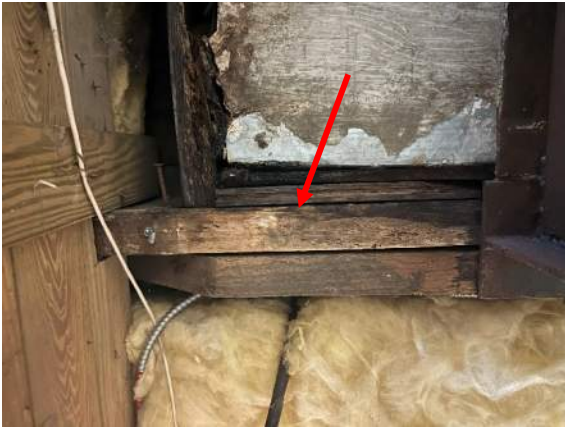
Picture 7 – Example of deteriorated beam at front side of deteriorated rim (pic 6)
