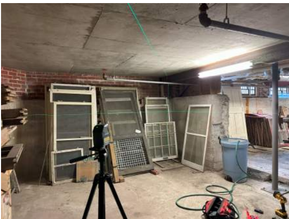
Picture 11 – Example of laser level set up for measurement of existing beams and underside of patio slab
