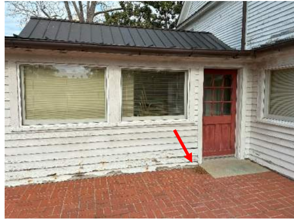
Picture 8 – Example of debris pile as evidence of previously standing water
