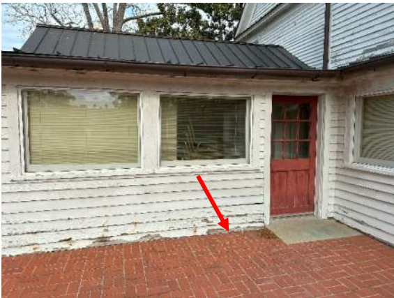
Picture 3 – Example of area of reported water- intrusion
