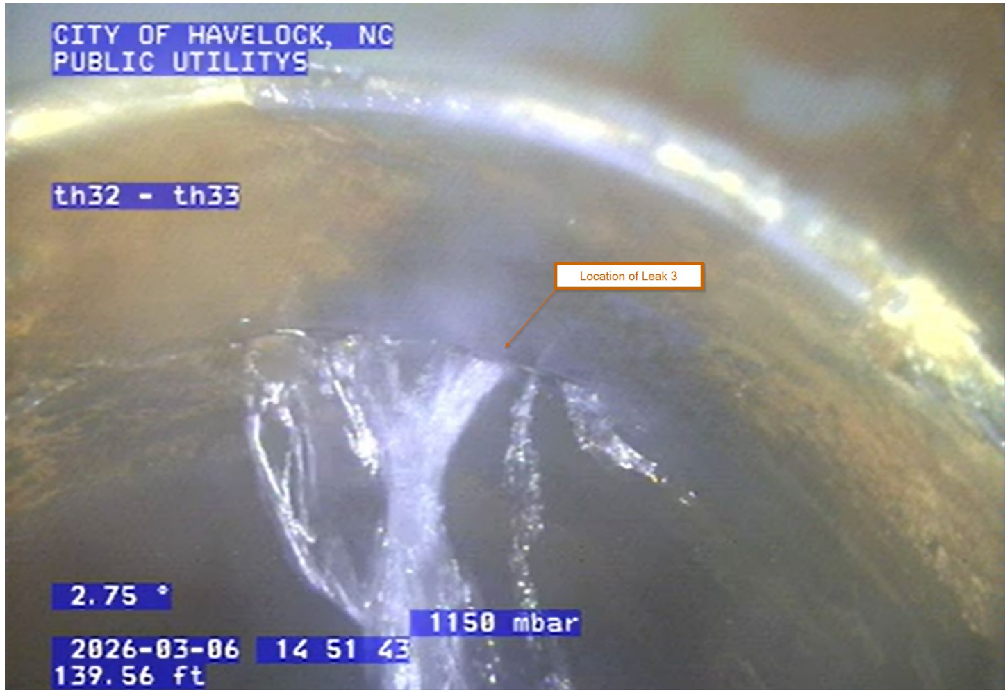
Figure 3: Forest Hill Leak 3
