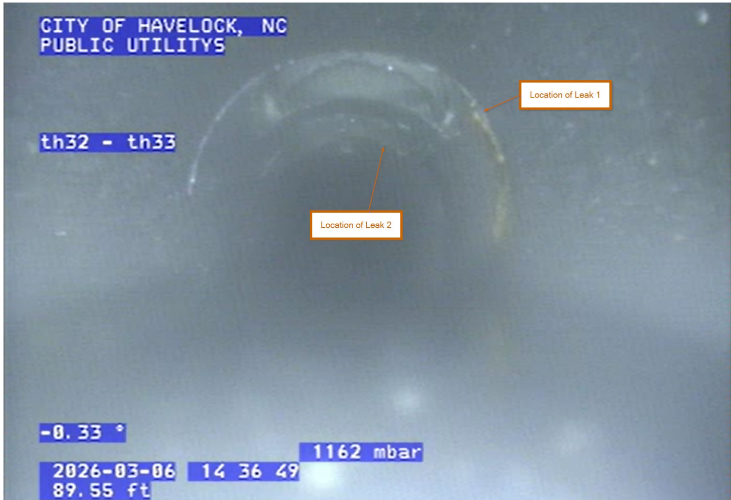
Figure 2: Forest Hill Leaks 1 and 2
