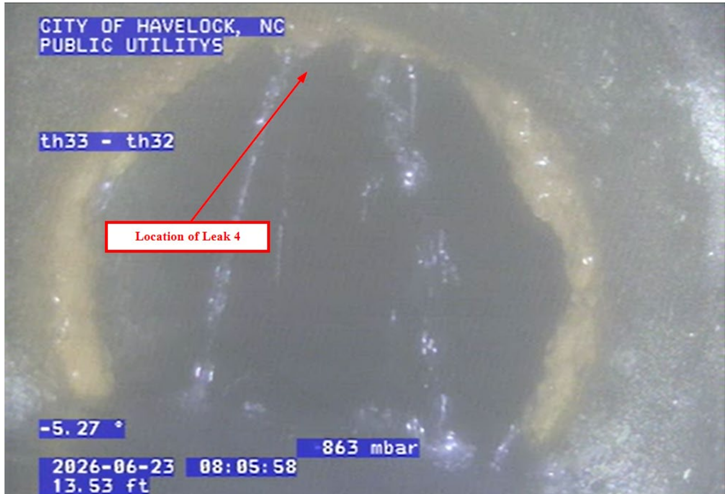
Figure 4: Forest Hill Leak 4
