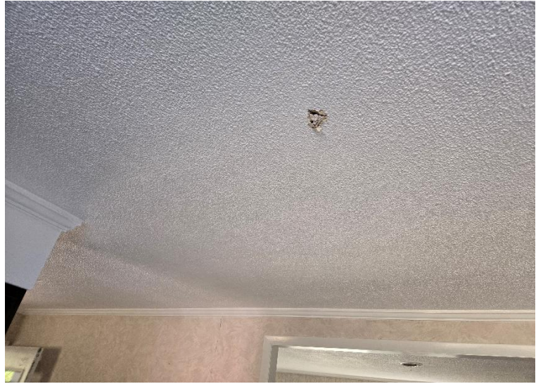
2. Kitchen Ceiling. Sample A-1
