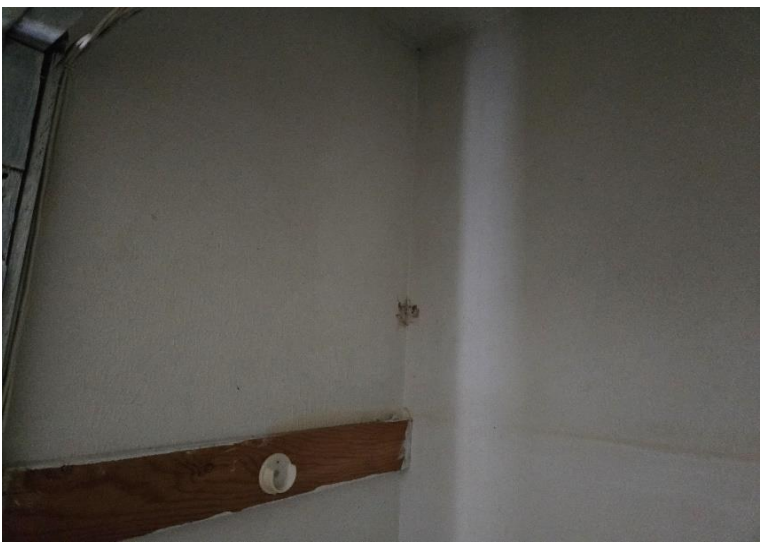
4. Closet Wall. Sample A-7
