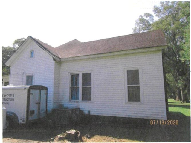
Unstable foundation supports.
