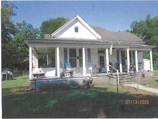
Major roof sagging.
