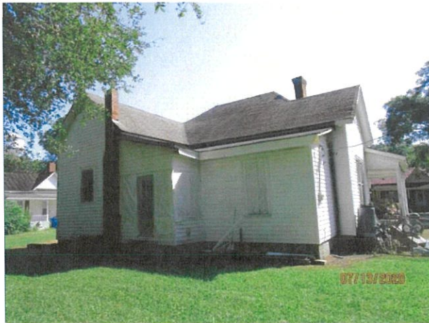
Exterior walls not weather-tight
