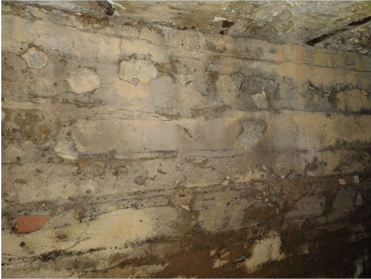
Figure 2. Typical Masonry Wall for Worth Box. Encased Steel Beams in Top ab visible above.
