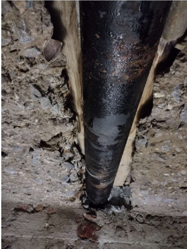
Figure 7. Embedded DIP in top slab of Worth St box with visible wood.
