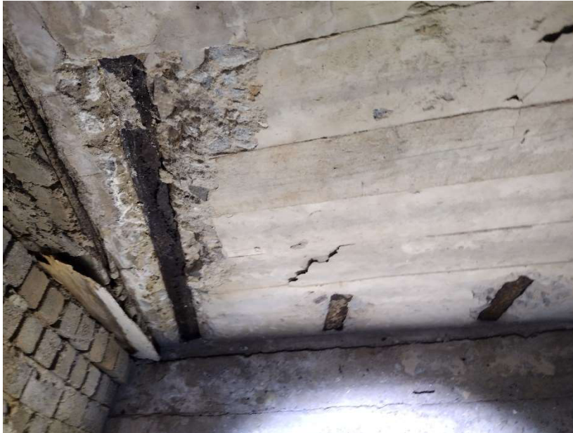
Figure 10. Partially exposed steel beams in Bloodworth junction box top slab & showing better condition of top slab compared to Worth St
