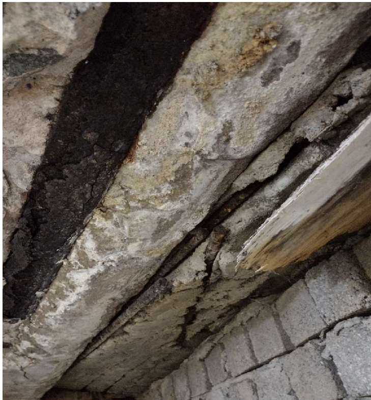
Figure 14. Exposed, unspliced reinforcement at one end of Bloodworth St junction box at transition of original top slab to newer RCP end wall.
