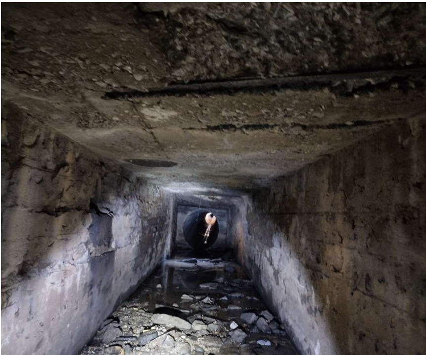
Figure 4. Interior view of Worth St box showing floor, walls, and top slab.
