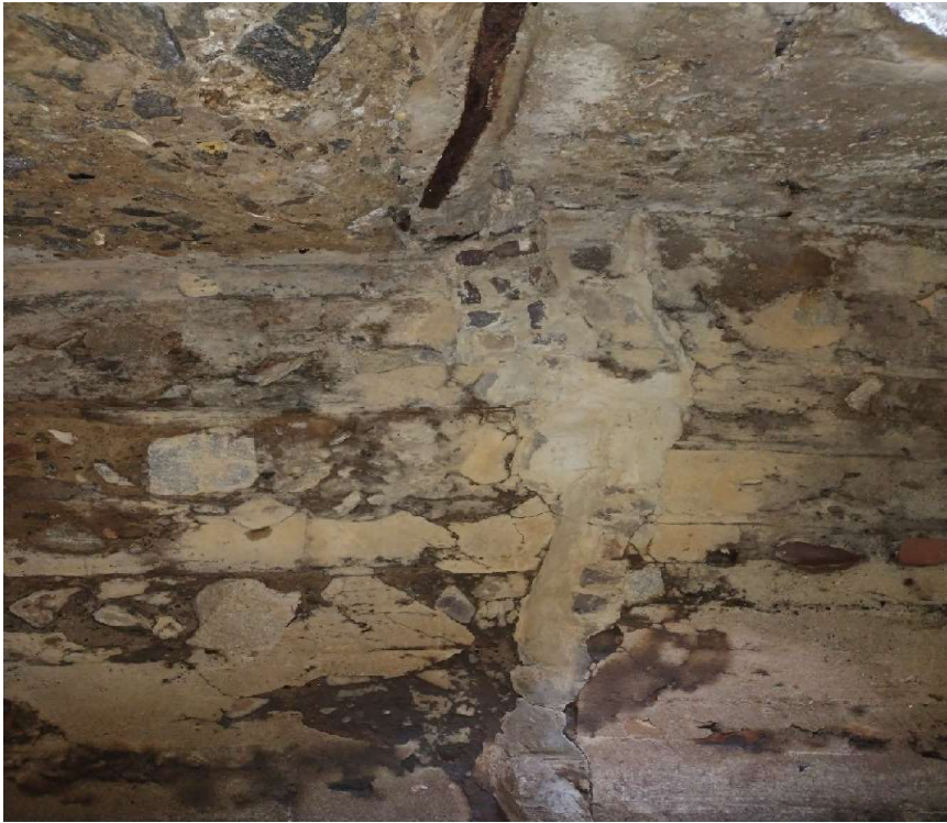
Figure 3. Repaired crack in box wall. No evidence of leaking or continued movement were observed.
