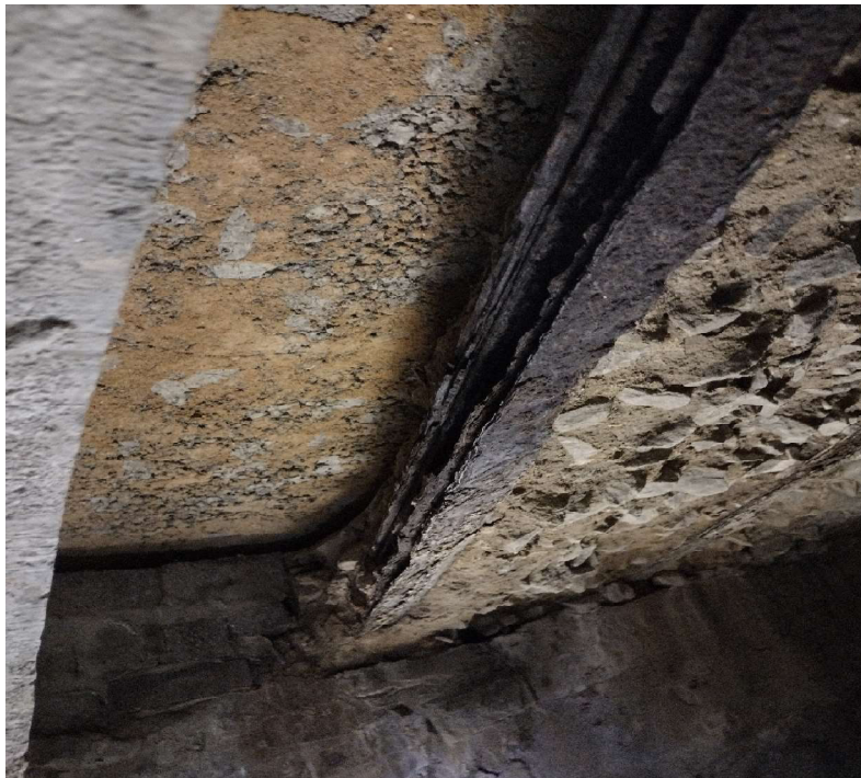
Figure 8. Comparison of original top slab concrete and the more recently placed concrete for the RCP end wall interface.
