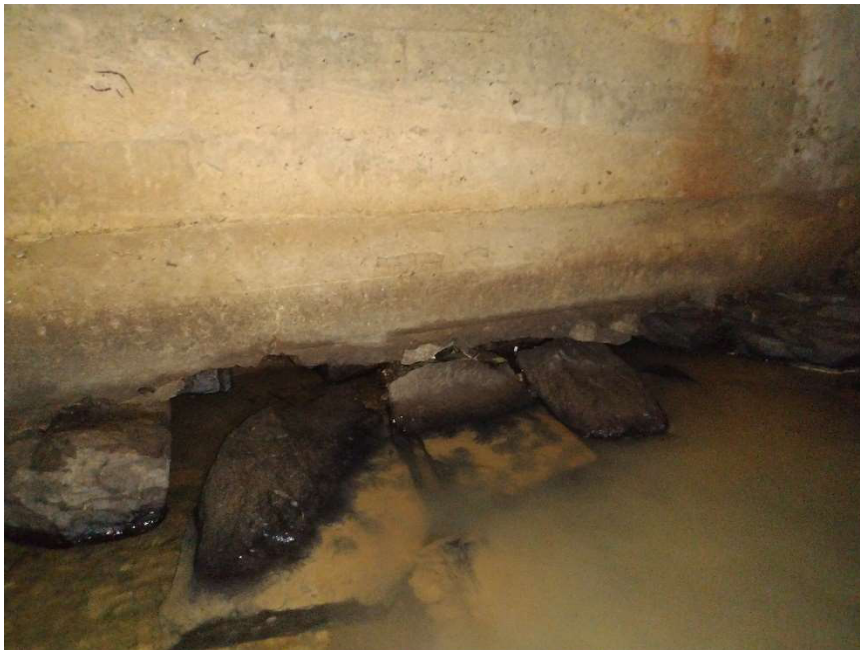
Figure 12. Noticeable void below the wall of Bloodworth junction box wall.
