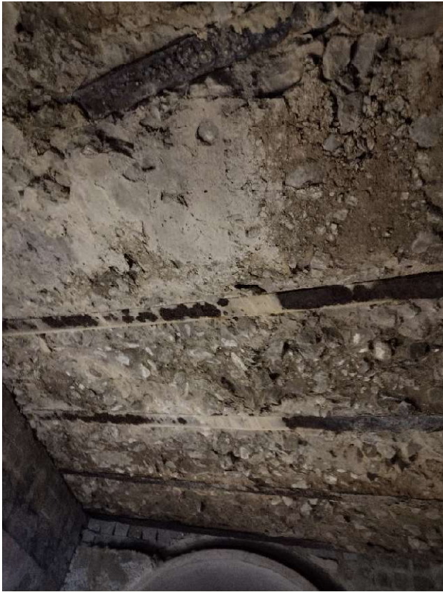
Figure 5. View of degradation on bottom of top slab at end of Worth St box.
