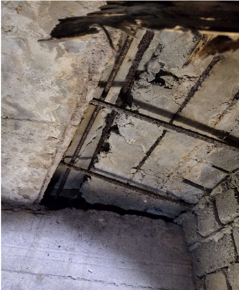
Figure 15. Exposed reinforcement at one end of Bloodworth St junction box at transition of original top slab to newer RCP end wall.
