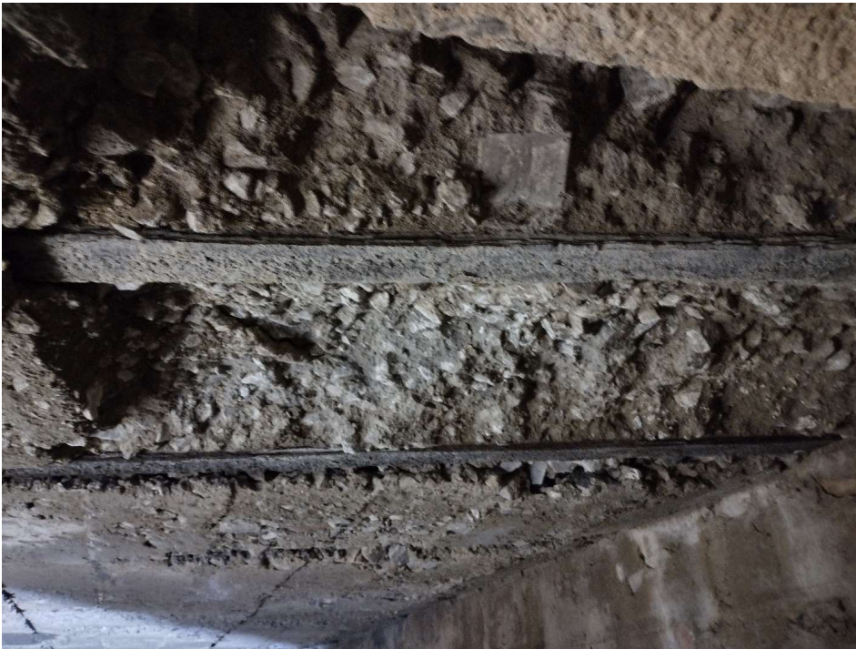
Figure 6. Visible steel corrosion and section loss of concrete between beams.
