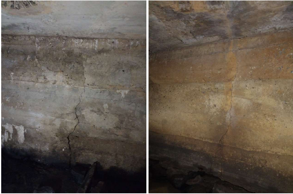
Figure 11. Unrepaired vertical cracks in wall of Bloodworth junction box
