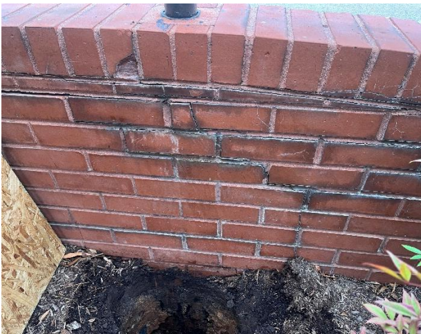
Photo 4 – Cracking along South Ramp Wall
