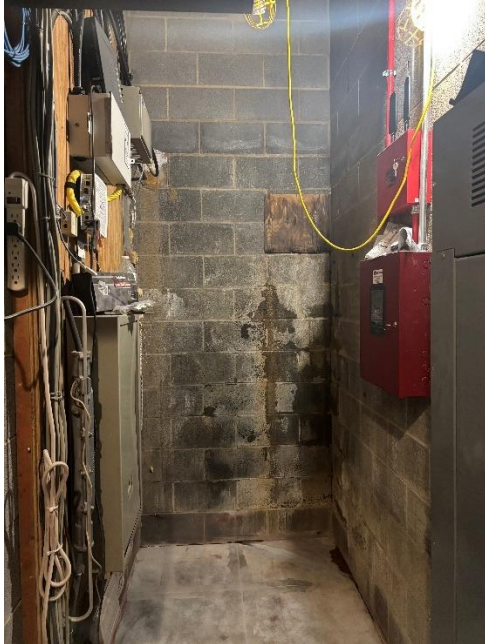
Photo 2 – Water Intrusion at SE Corner
