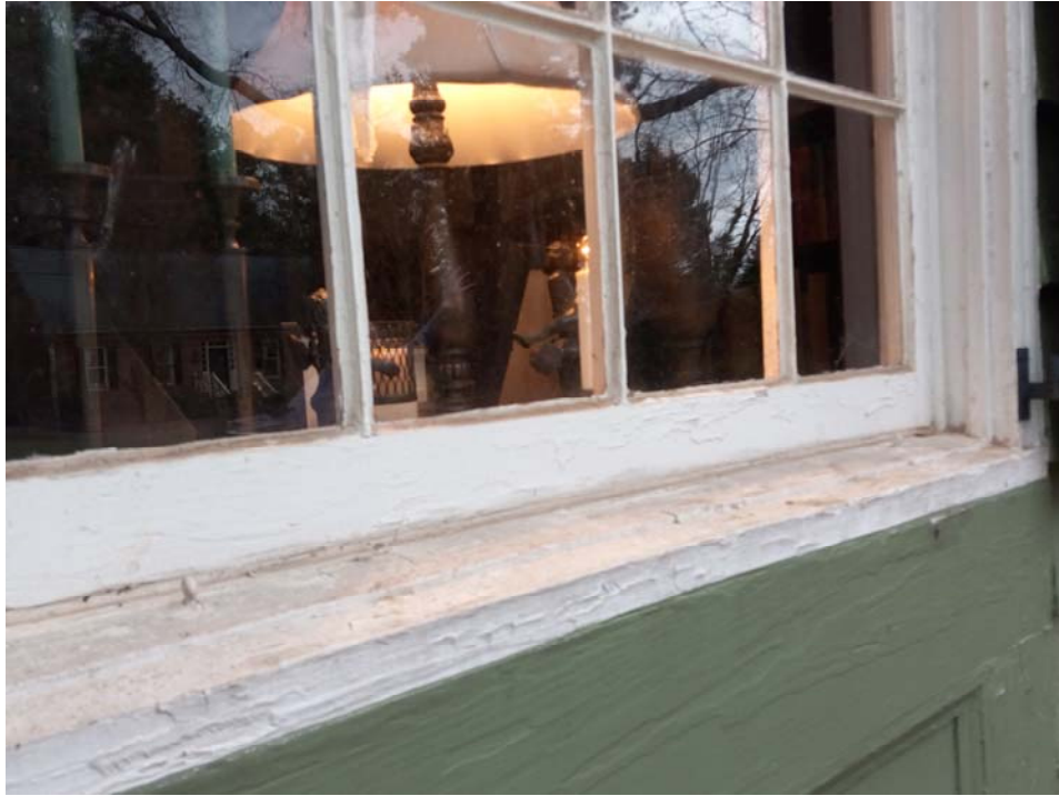
Photo #5: Peeling Exterior Window Components
