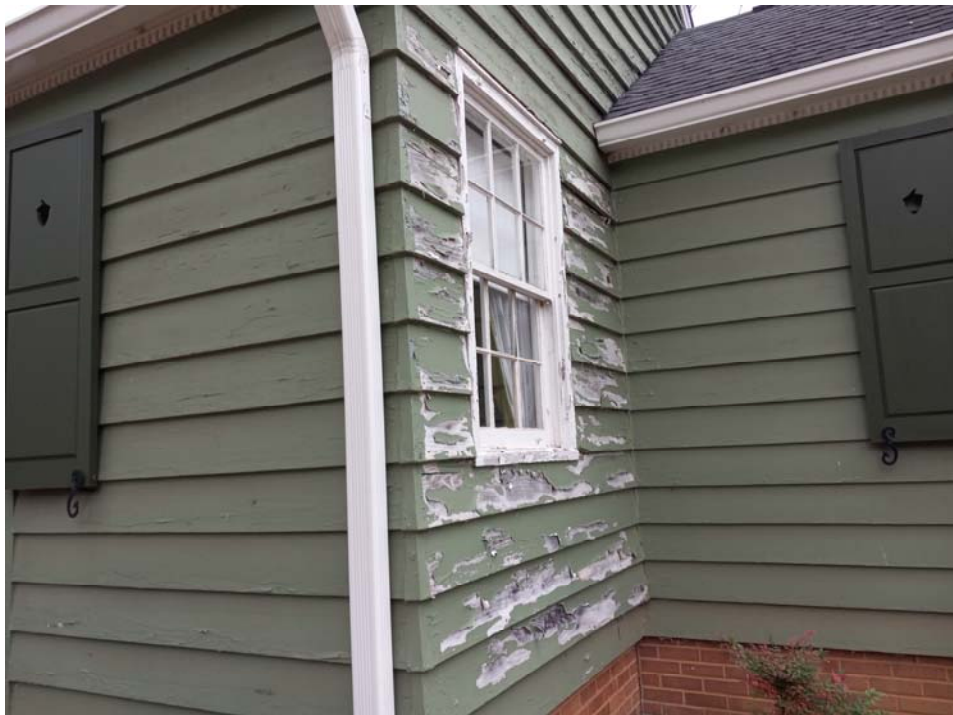
Photo #6: Peeling Siding
