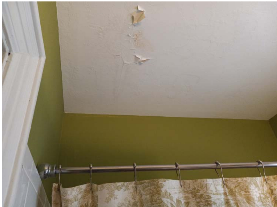
Photo #4: Peeling Paint – Bathroom Ceiling
