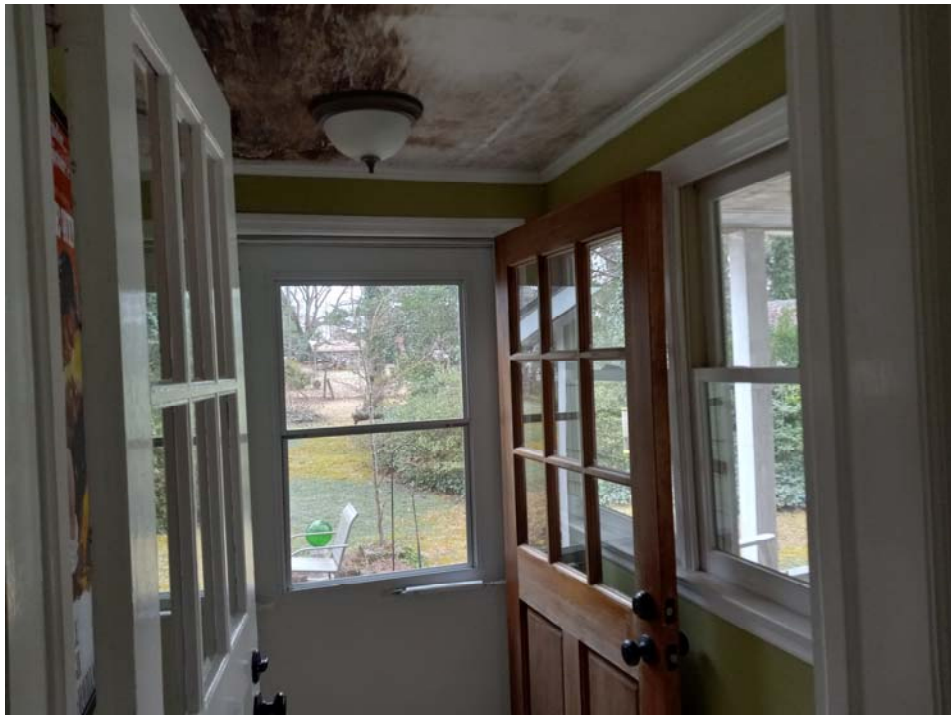
Photo #2: Mudroom Damaged Ceiling
