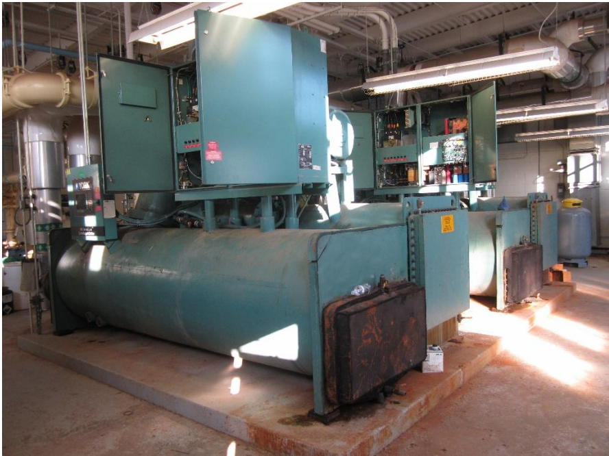
Photo: water cooled chiller inside Chiller Plant
