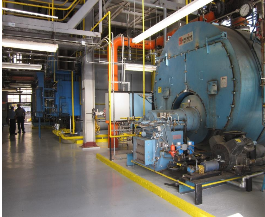
Photo: fire tube steam boiler (800 hp) inside of Steam Plant Building
