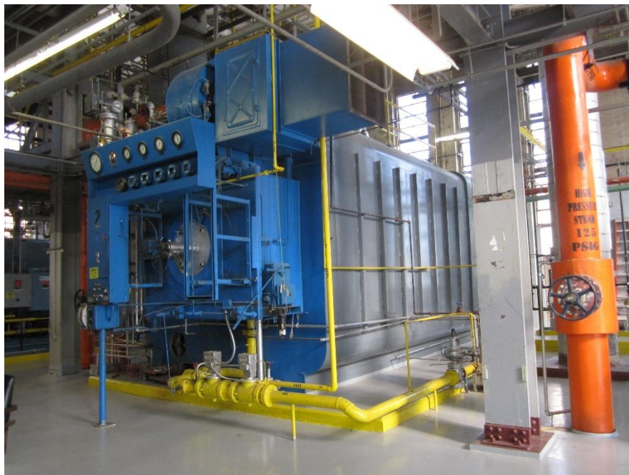
Photo: water tube steam boiler (1500 hp) inside of Steam Plant Building
