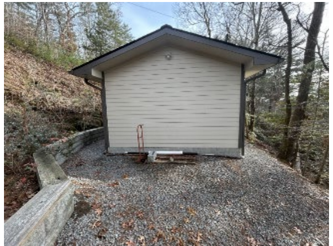
Garage and landslide
