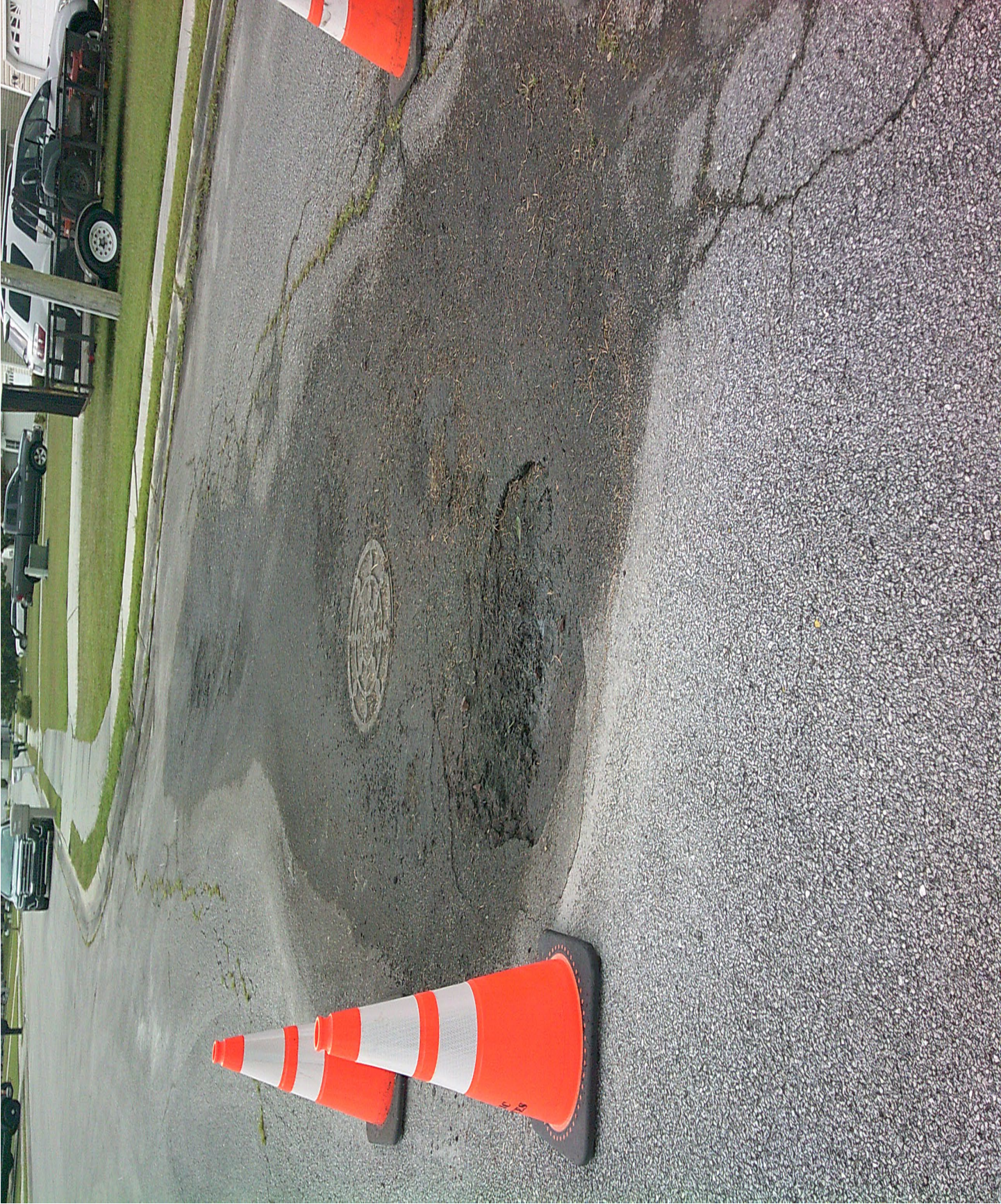
Figure 7: Image of the sinkhole.
