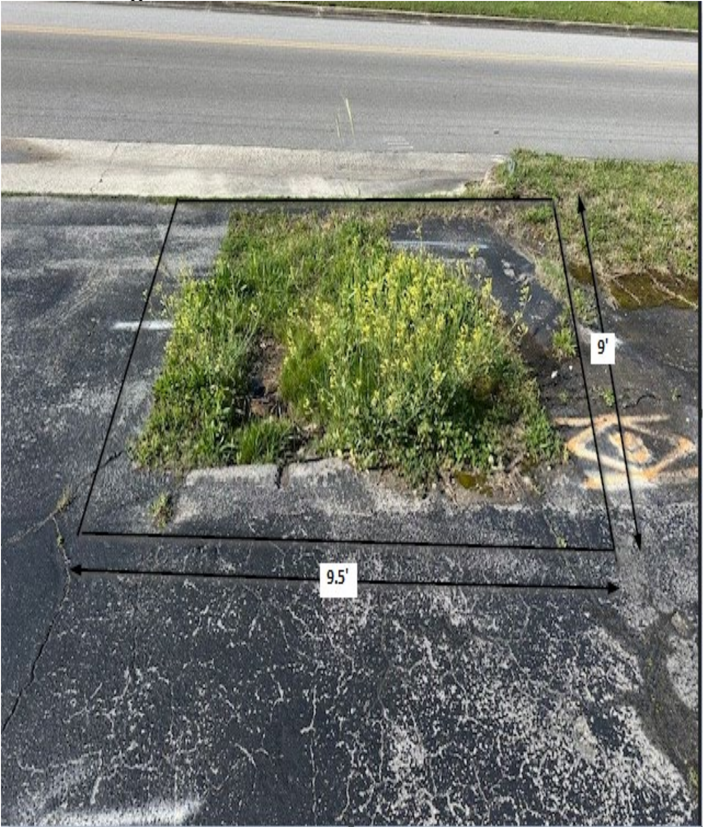
Figure 29: 112 W. Main St. / Area F / This area shall be cut square before repairing the utility cut. Measurements are approximate.
