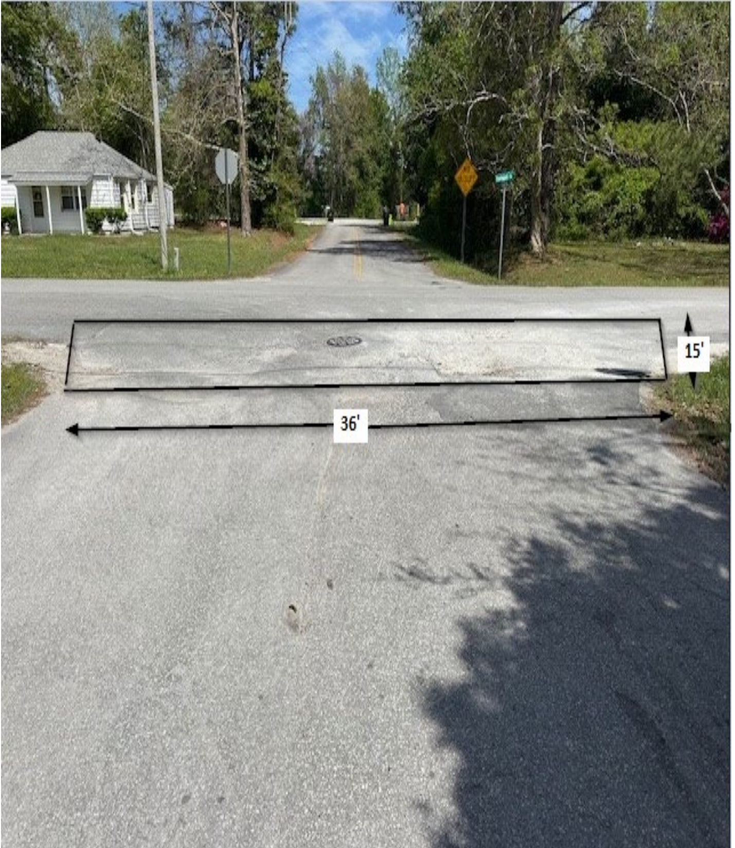
Figure 3: Fleetwood and Carolina / Area A / This area shall be cut square before repairing the utility cut. Measurements are approximate.
