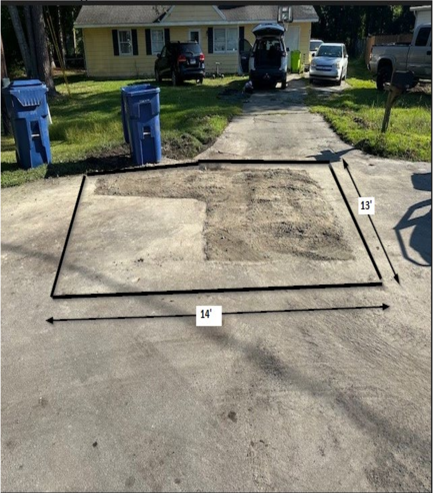
Figure 27: 508 Blarney / Area D / This area shall be cut square before repairing the utility cut. Measurements are approximate.
