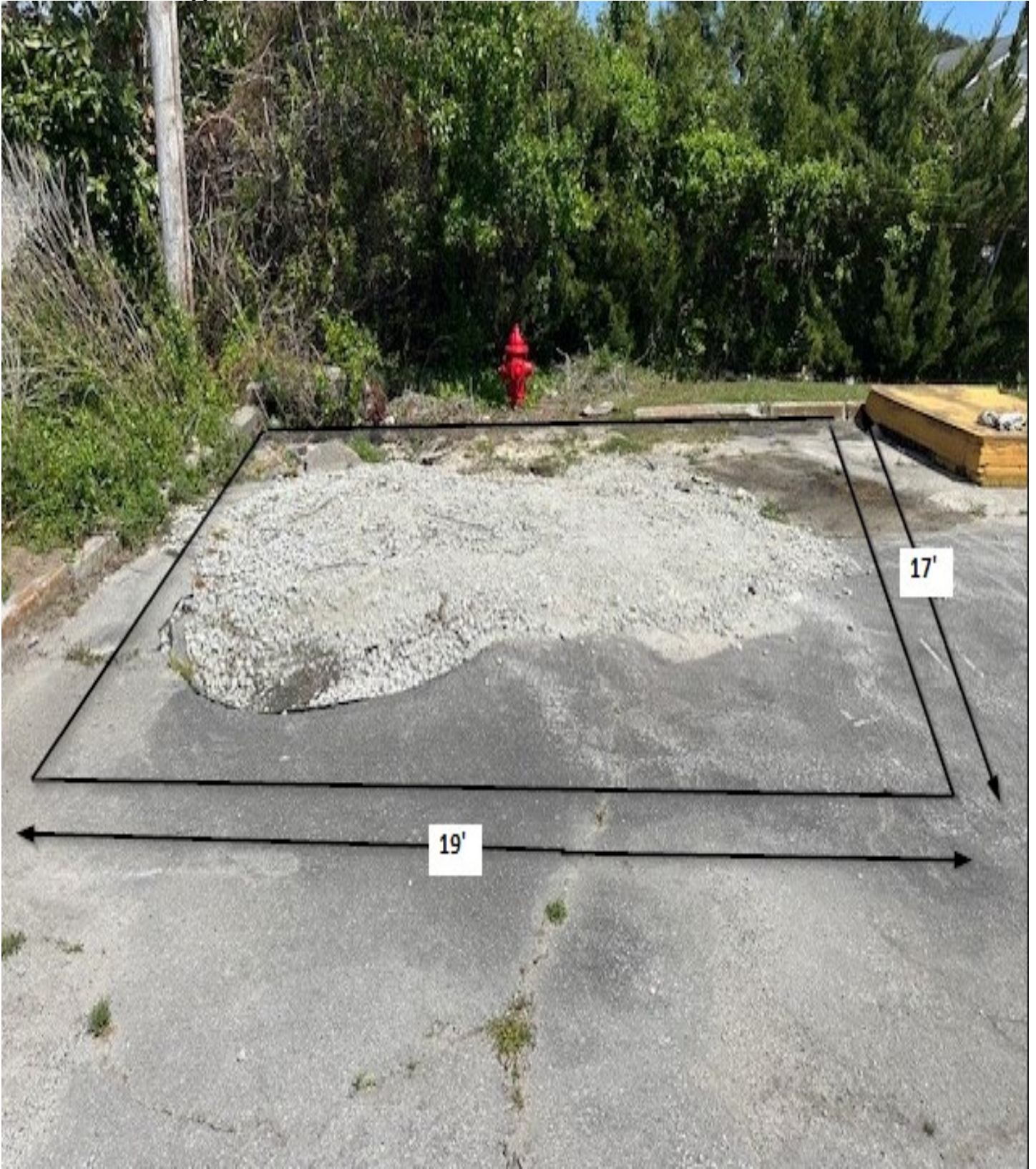
Figure 18: 1313 E. Main St. / Area A / This area shall be cut square before repairing the utility cut. Measurements are approximate.
