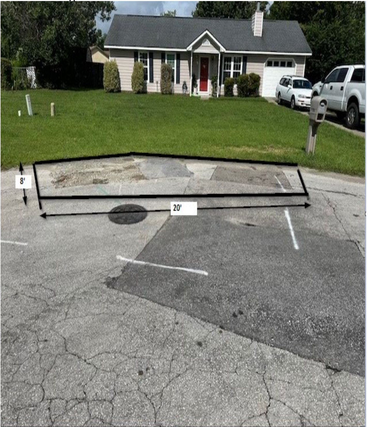
Figure 14: 401 Cottonwood / Area A / This area shall be cut square before repairing the utility cut. Measurements are approximate.
