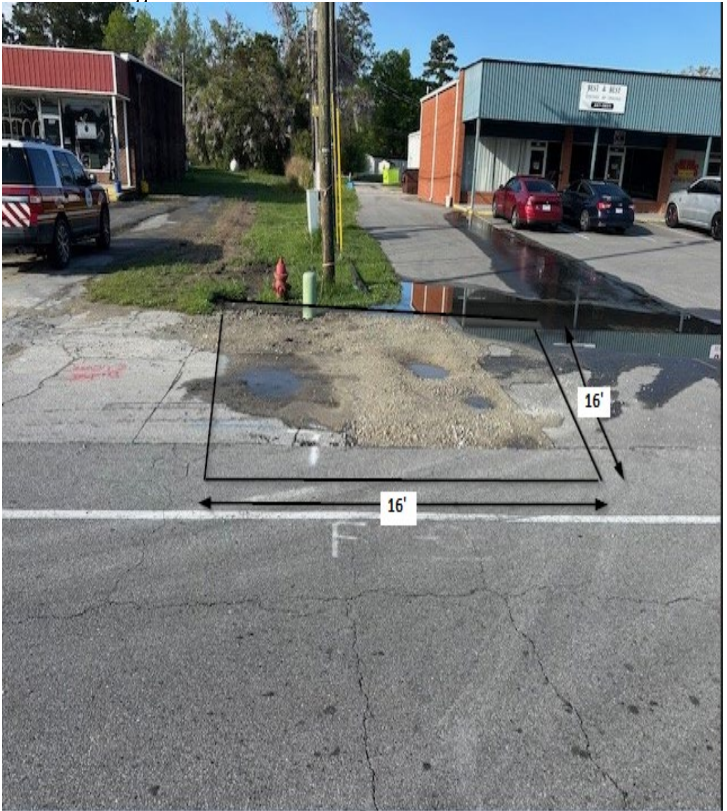
Figure 30: 309 W. Main St / Area F / This area shall be cut square before repairing the utility cut. Measurements are approximate.
