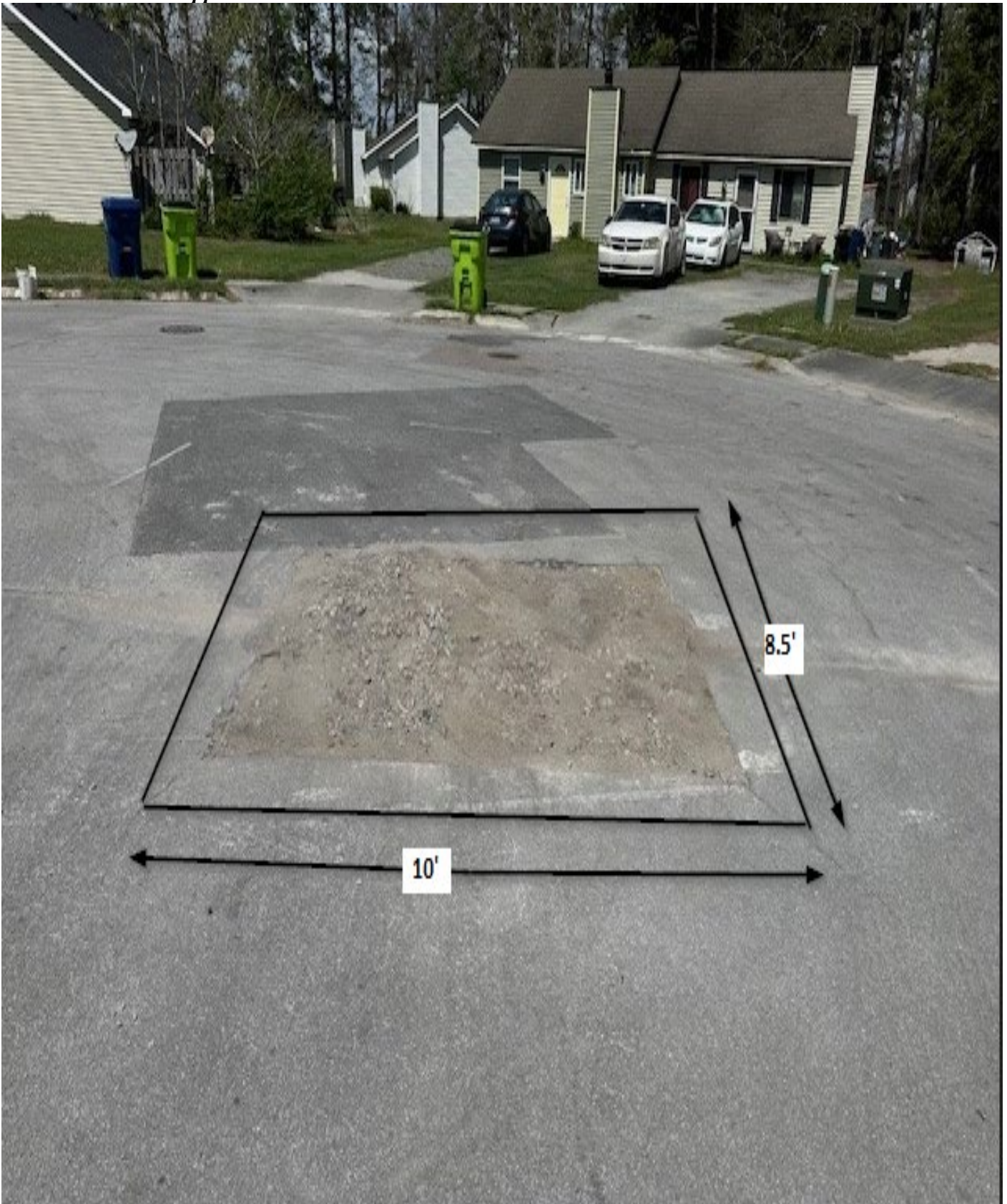
Figure 20: 208 Cedar Ridge Ct. / Area A / This area shall be cut square before repairing the utility cut. Measurements are approximate.
