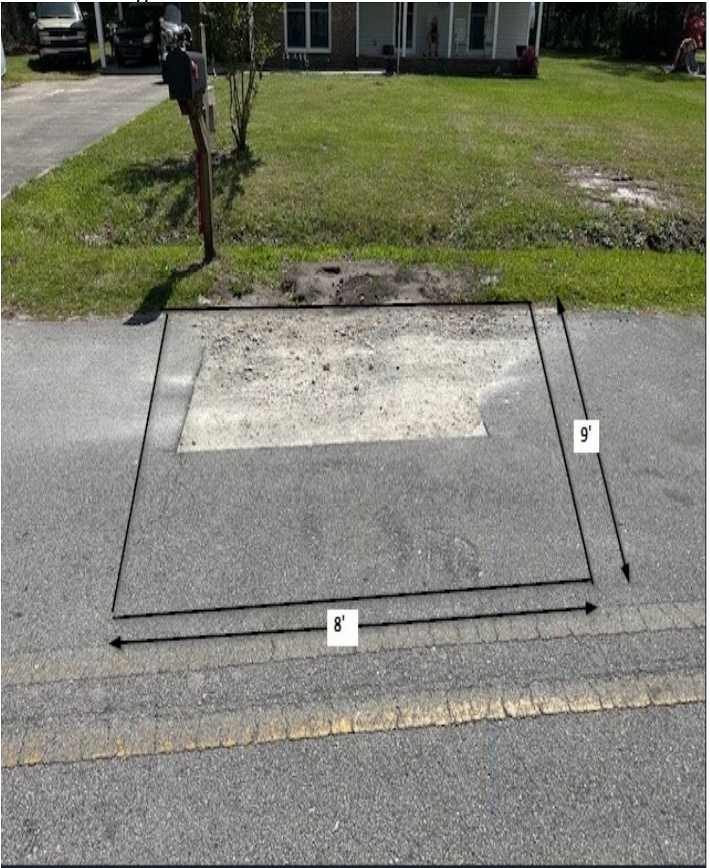
Figure 33: 203 Pineview / Area H / This area shall be cut square before repairing the utility cut. Measurements are approximate.
