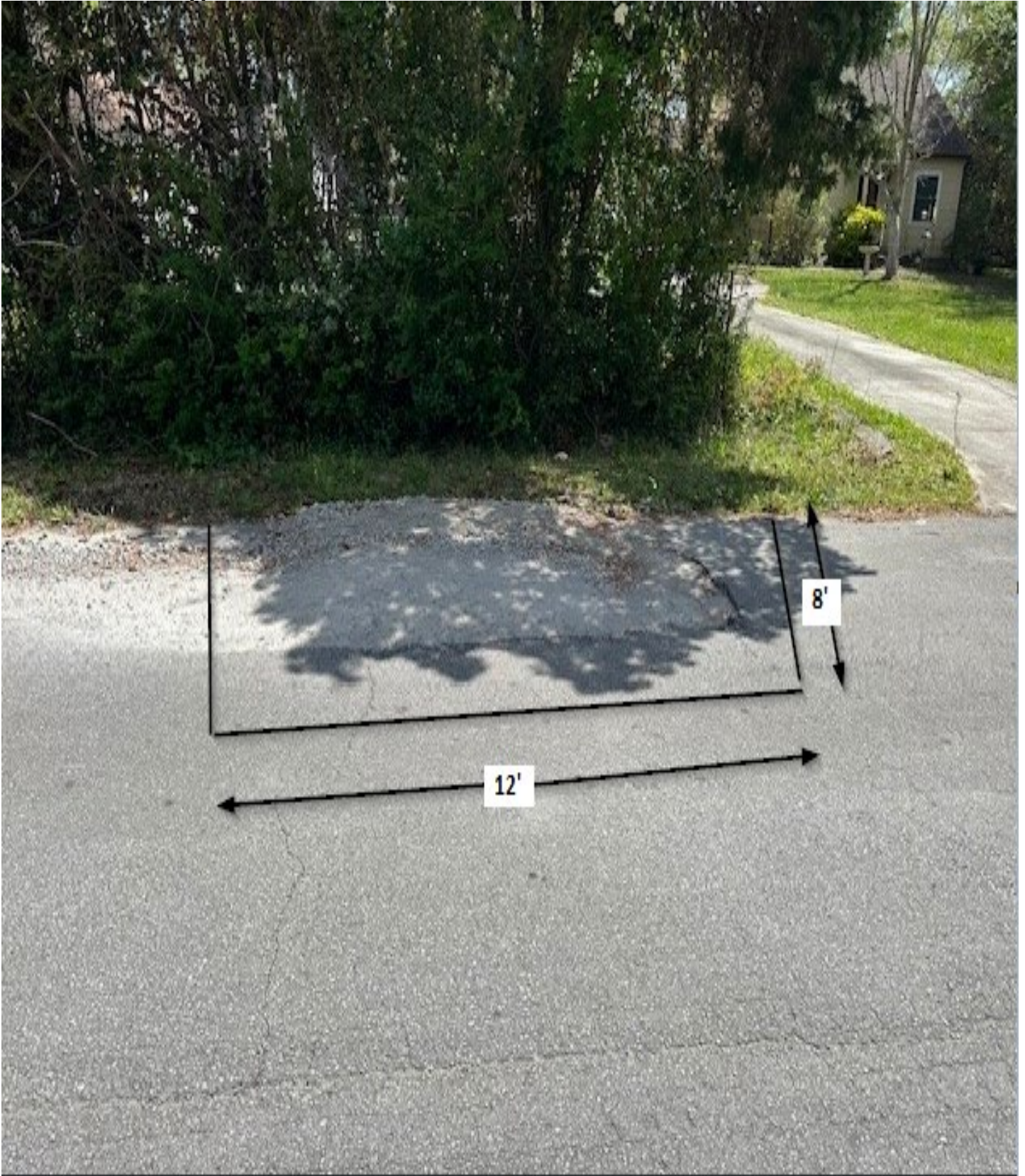
Figure 9: 110 Carolina / Area A / This area shall be cut square before repairing the utility cut. Measurements are approximate.
