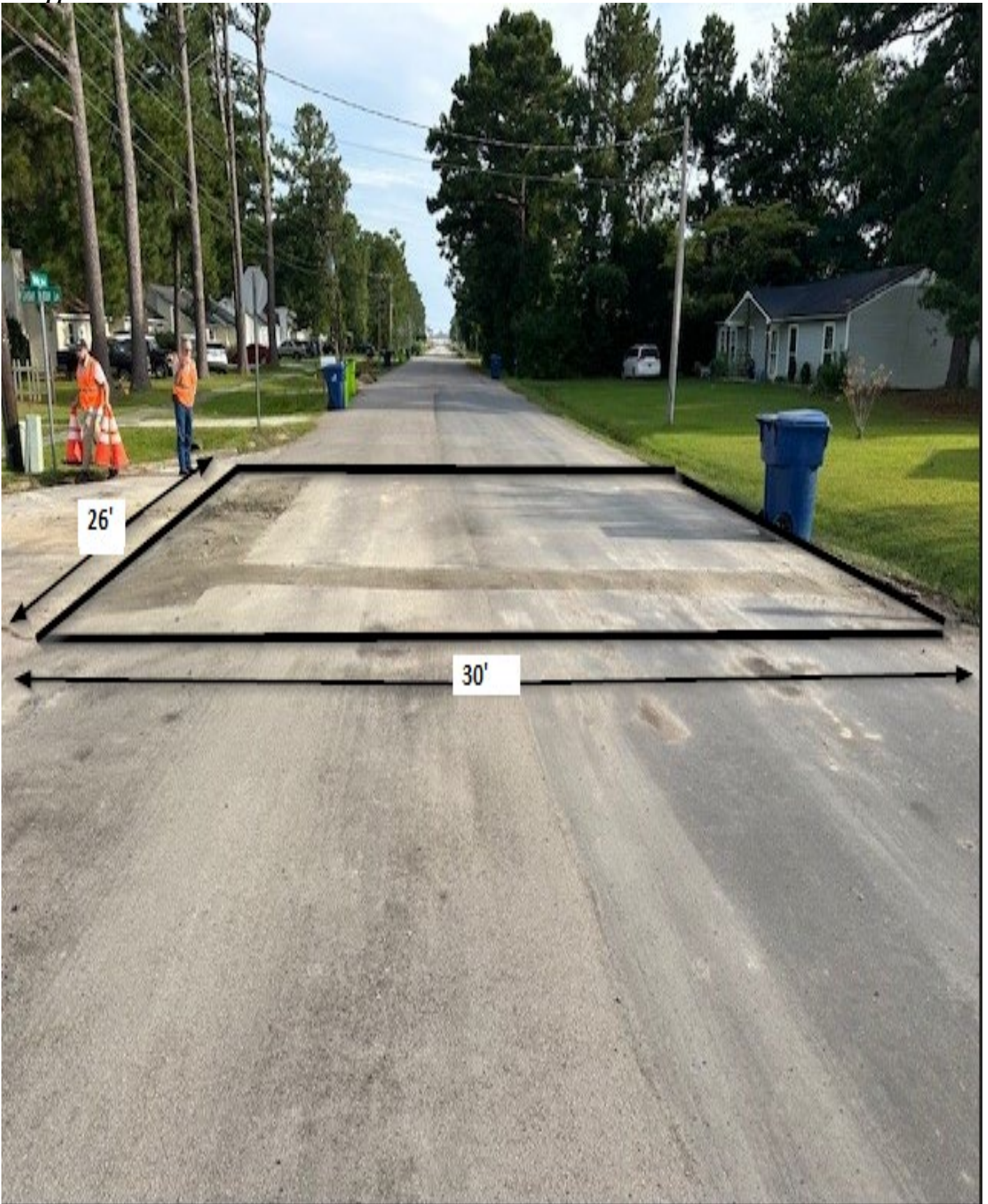
Figure 21: 203 Webb / Area A / This area shall be cut square before repairing the utility cut. Measurements are approximate.
