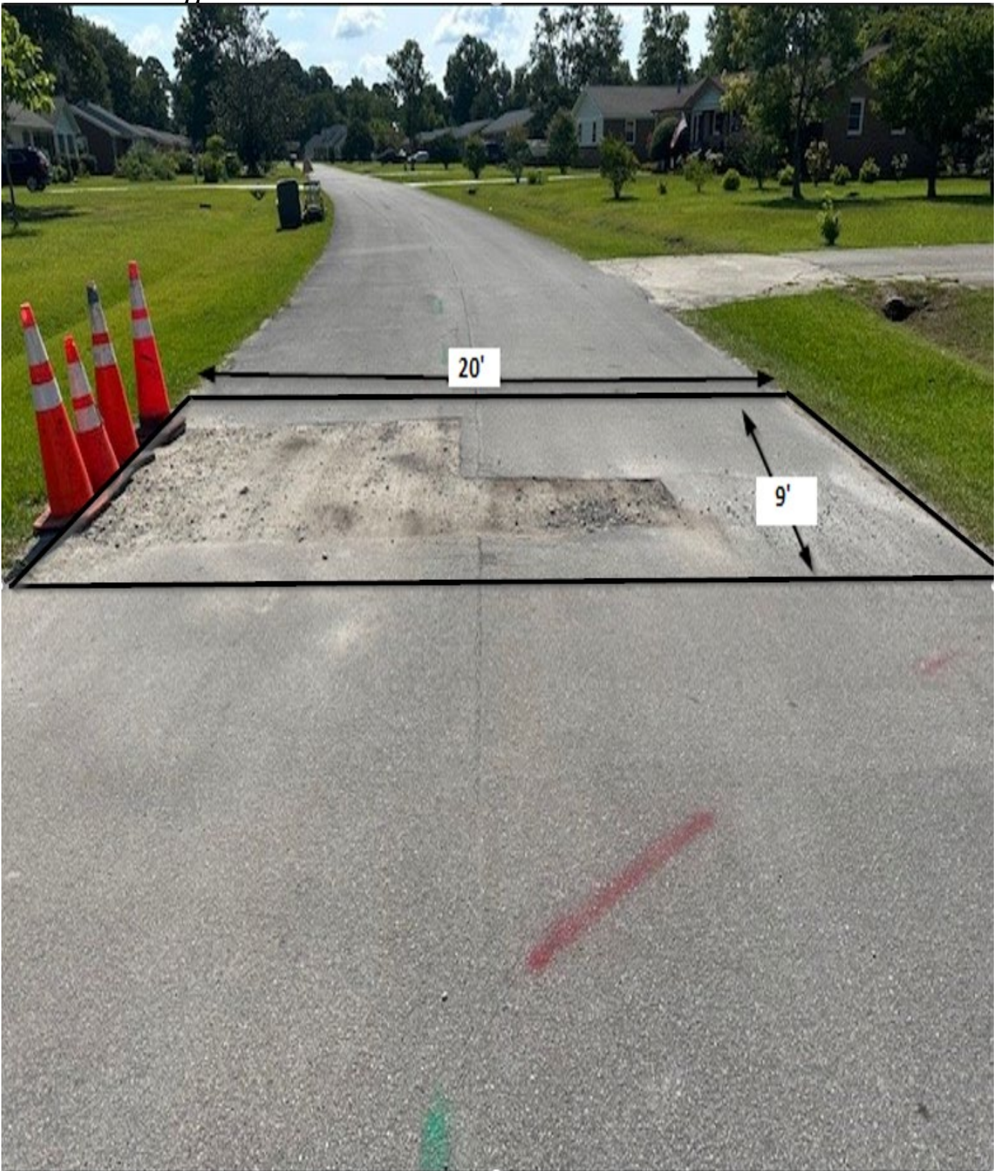
Figure 32: 120 Craven / Area H / This area shall be cut square before repairing the utility cut. Measurements are approximate.
