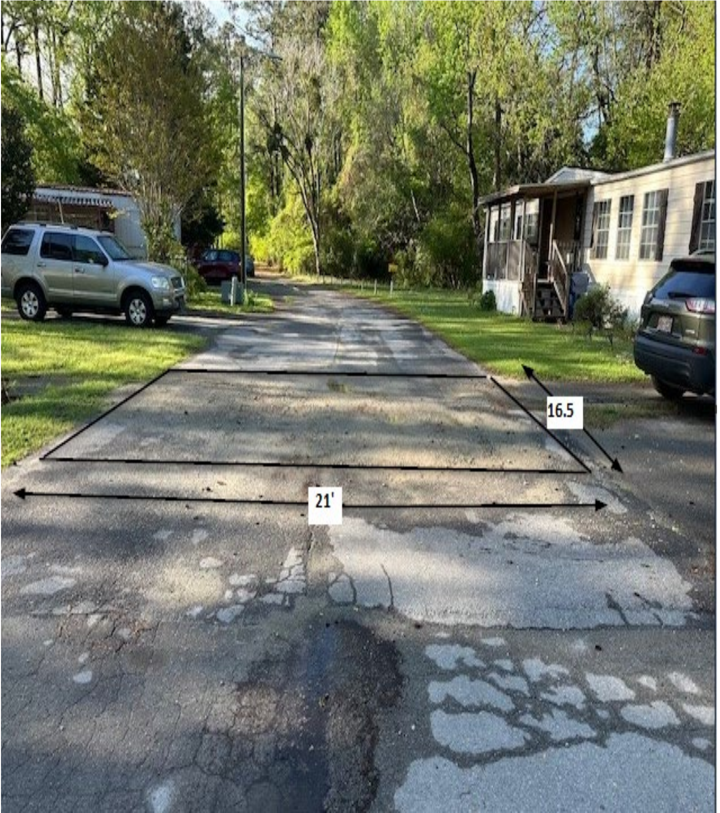
Figure 35: 228 Russel / Area J / This area shall be cut square before repairing the utility cut. Measurements are approximate.
