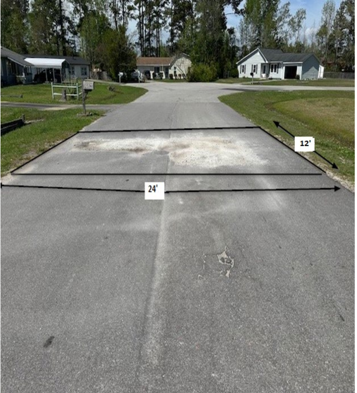
Figure 8: 107 Pirates / Area A / This area shall be cut square before repairing the utility cut. Measurements are approximate.
