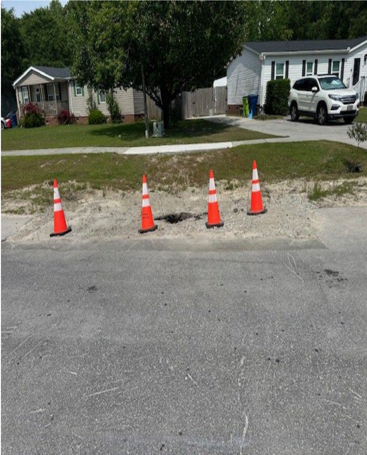
Figure 2: 321 Utility Cut and Sinkhole.
