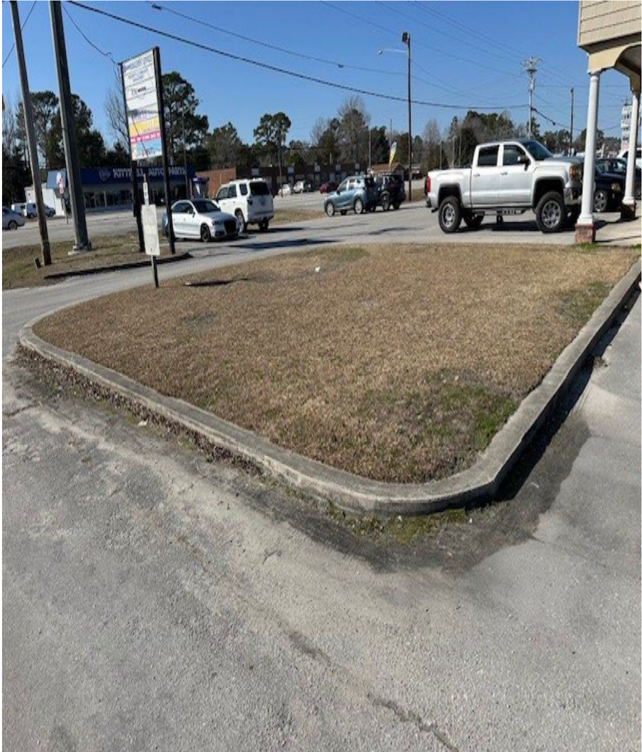
Figure 4: Curbing to be removed and replaced and raised grass island to be resodded after curbing restoration.
