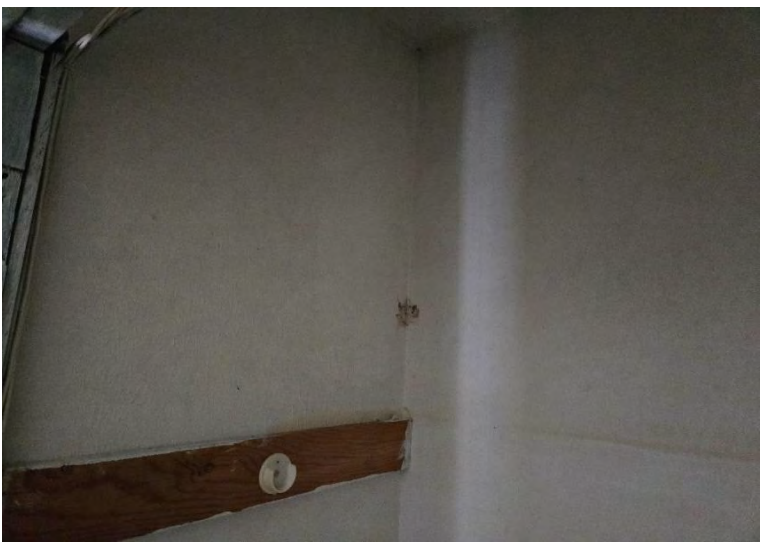
4. Closet Wall. Sample A-7
