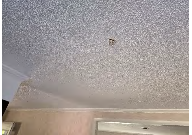
2. Kitchen Ceiling. Sample A-1
