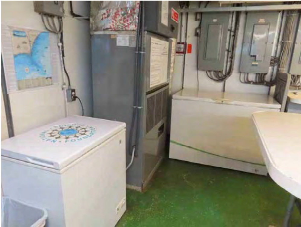
69. Freezer and AC unit
