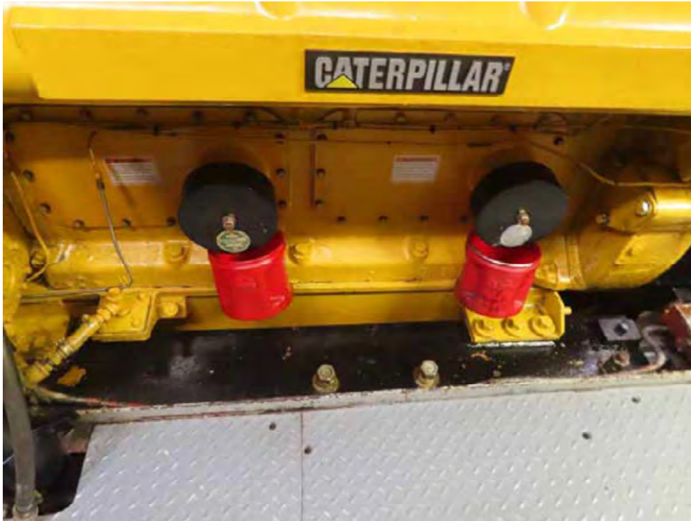
79. Small leaks on main engine
