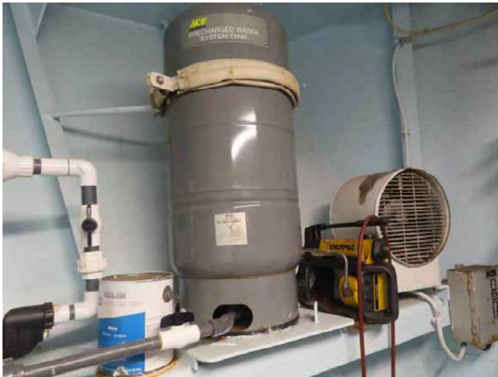
46. Pre-charged water system
