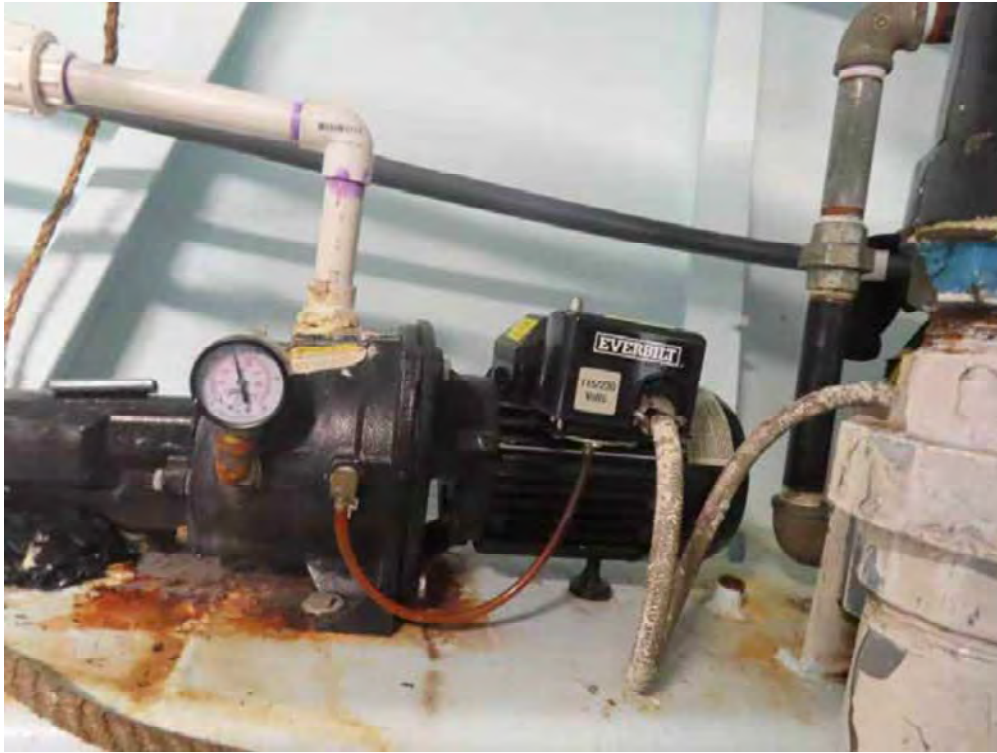
47. Fresh water pump
