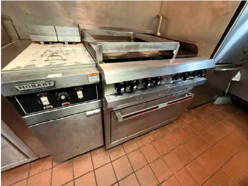
57. Main galley oven/cooktop and deep fryer (Fryer reportedly inoperative)
