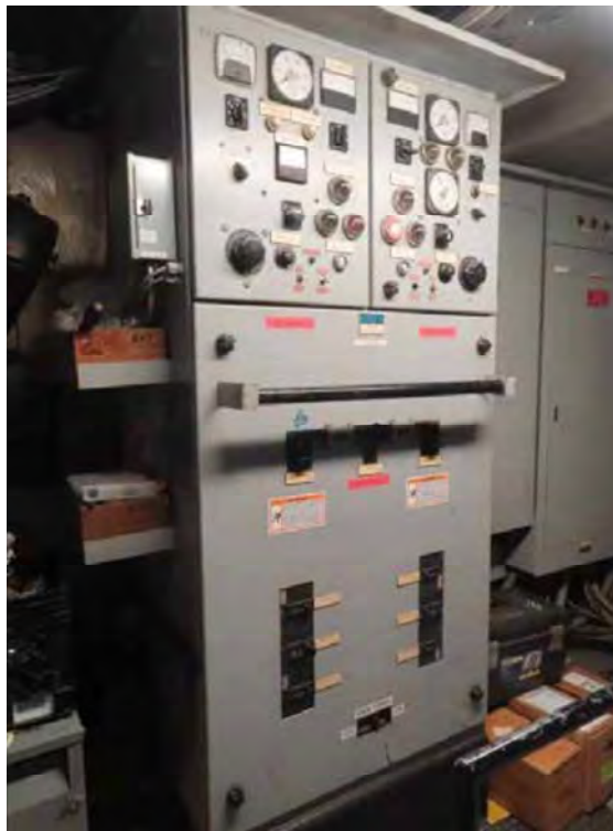
88. Electrical distribution panel in electrical room on main deck
