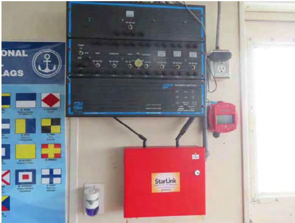
23. Starlink Fire Alarm Communicator
