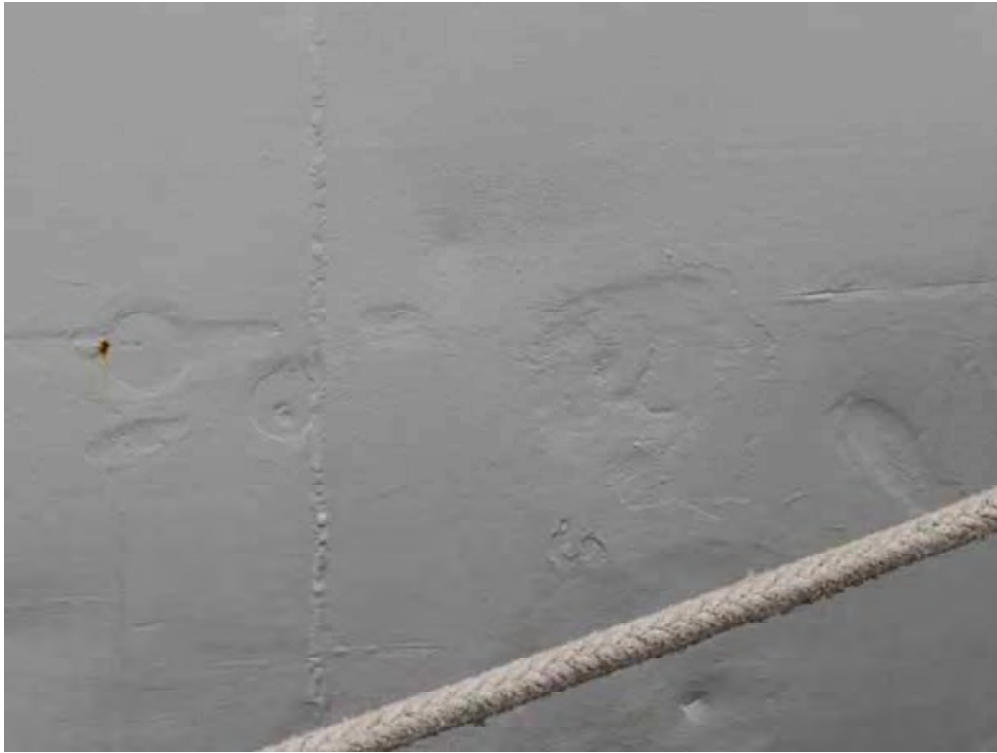
7. Signs of arrested pitting on starboard side
