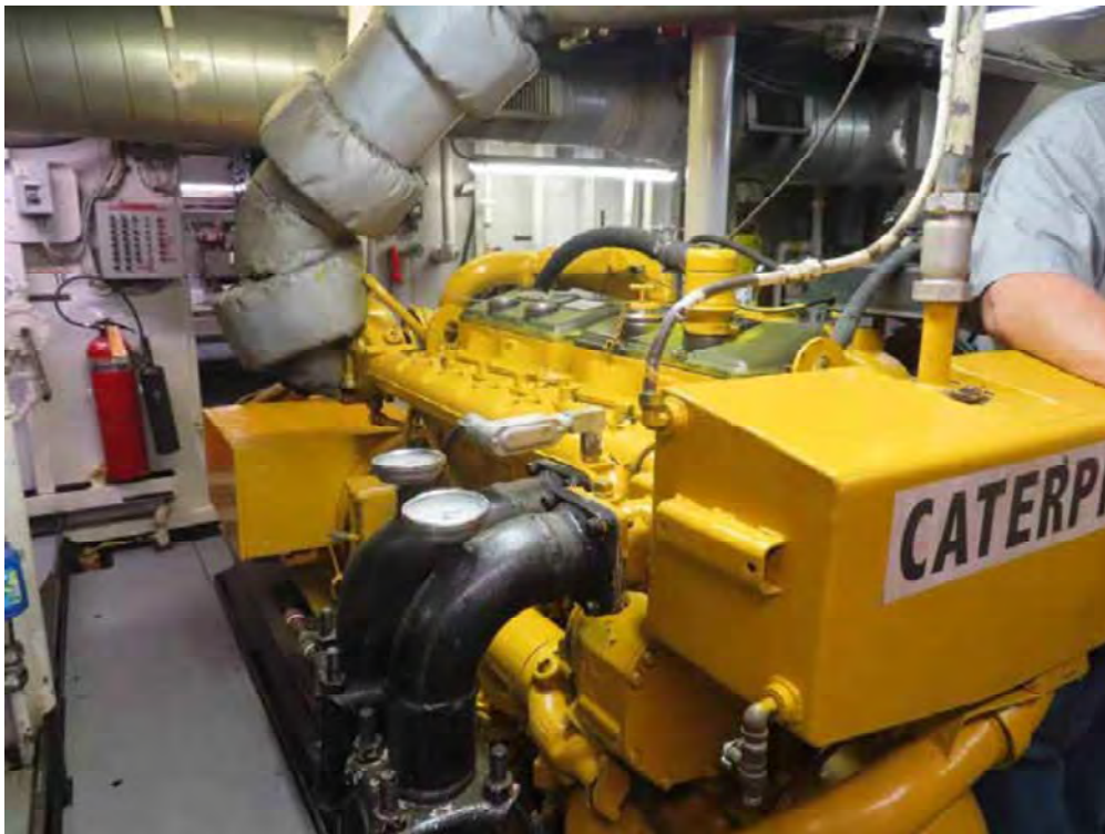
76. Starboard main engine
