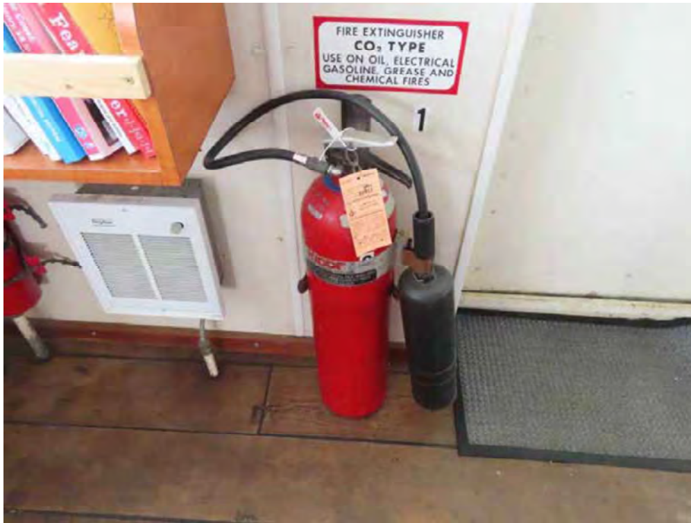
93. Typical CO2 portable fire extinguisher station
