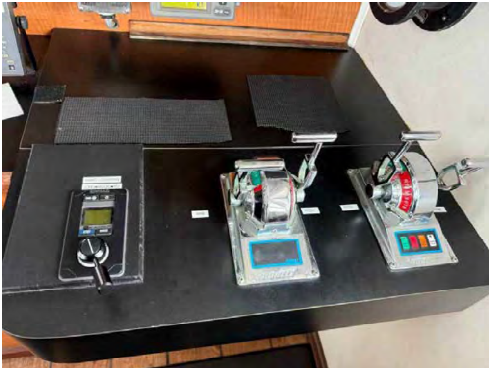
28. . Reversible pitch propeller pilot station with non-follow up rudder control starboard aft deck house
