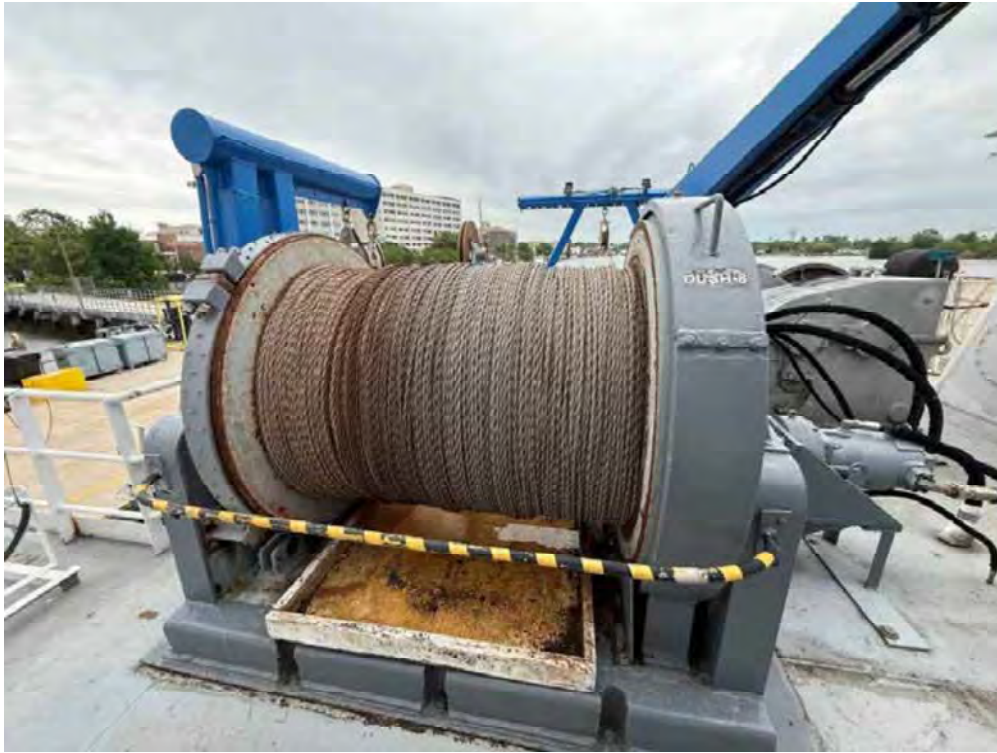
13. Main trawl winch on 01 level aft
