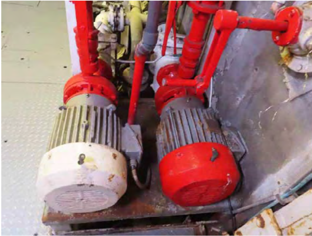
83. Bilge and fire pump
