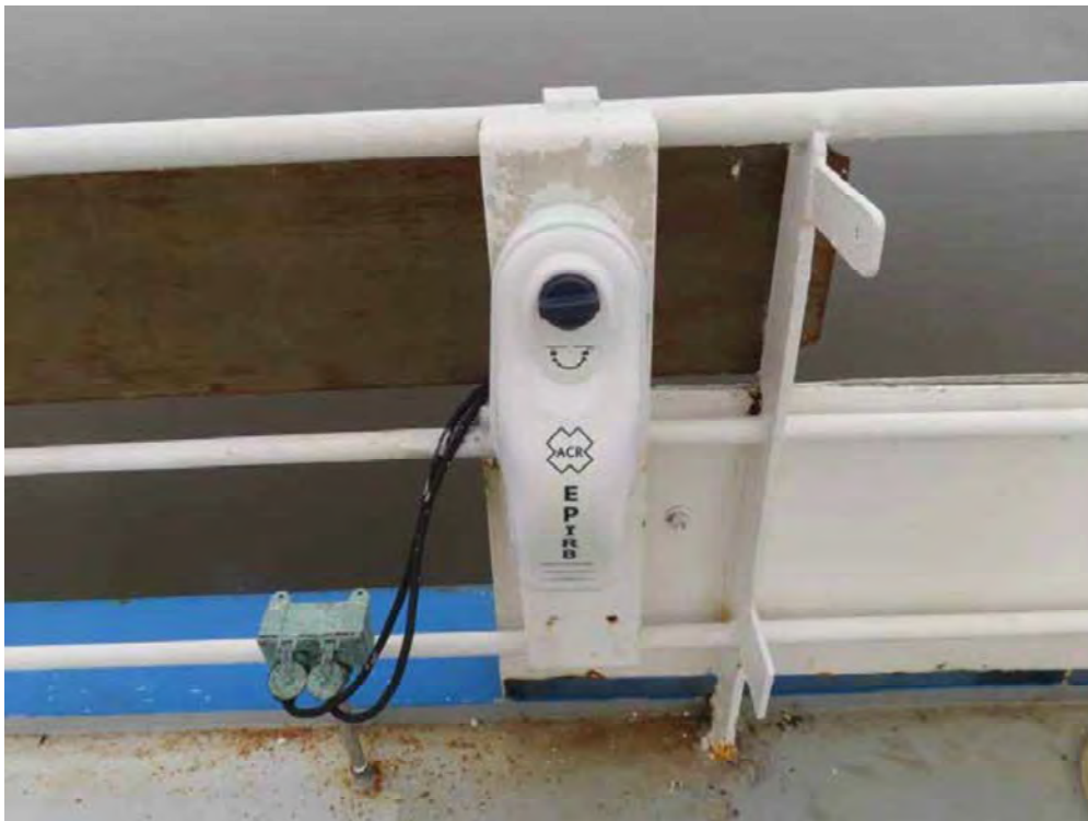
96. EP|IRB mounted on flying bridge
