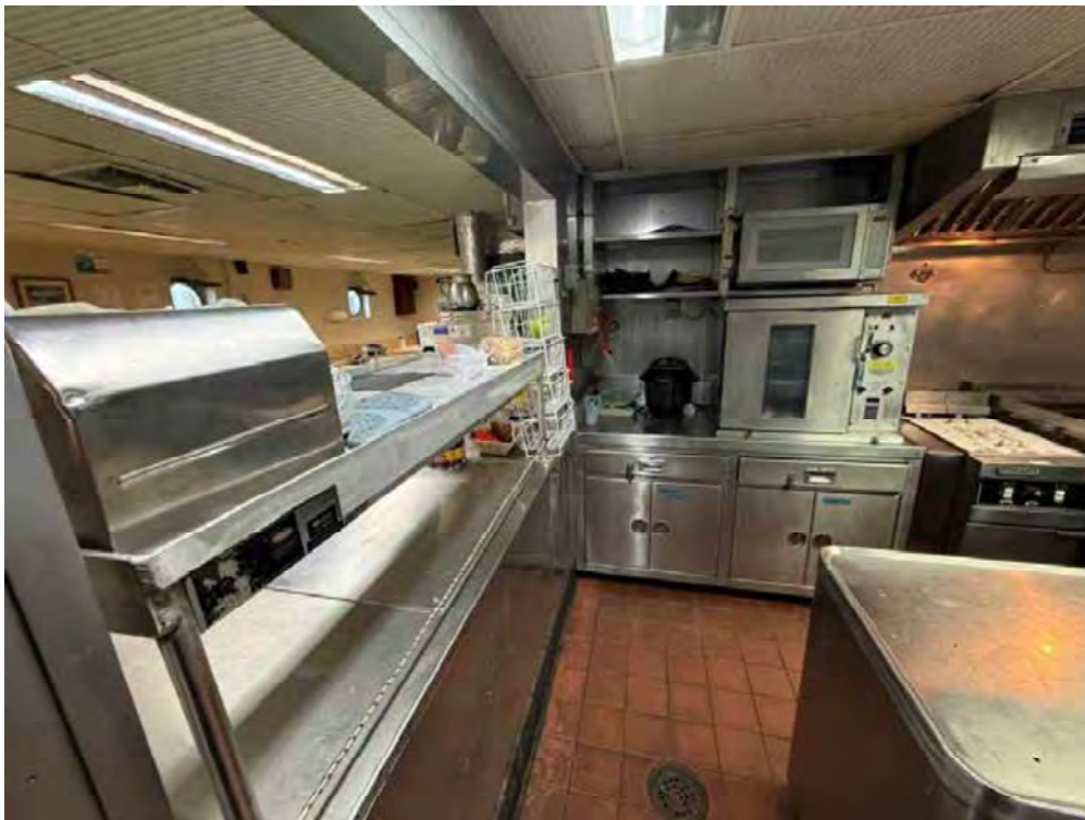
56. Main galley rack oven/microwave and cabinets
