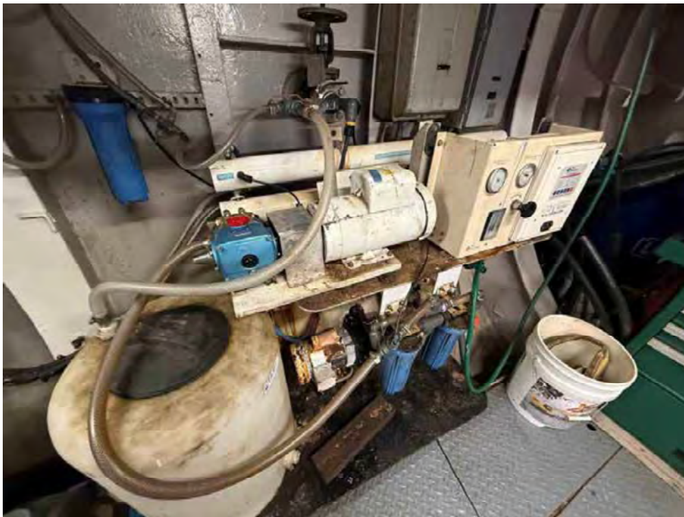
84. Fresh water maker system
