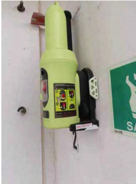
95. SART mounted on starboard side 01 level
