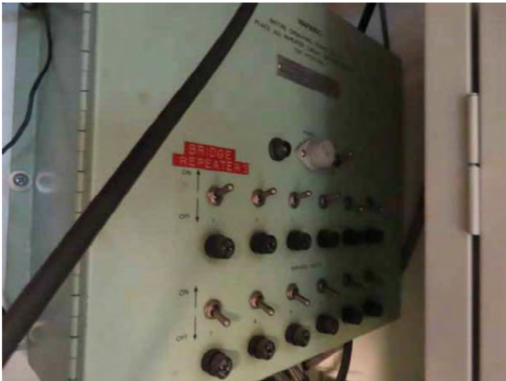
64. Gyrocompass control panel
