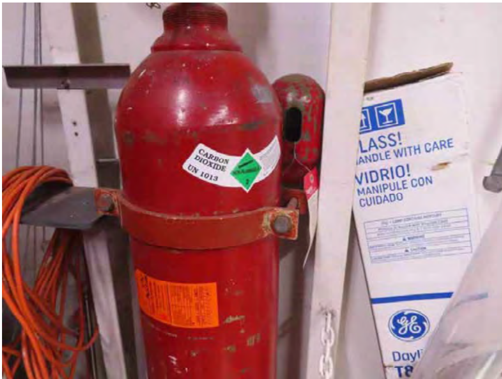
90. Fixed CO2 bottle for paint locker fire firefighting system
