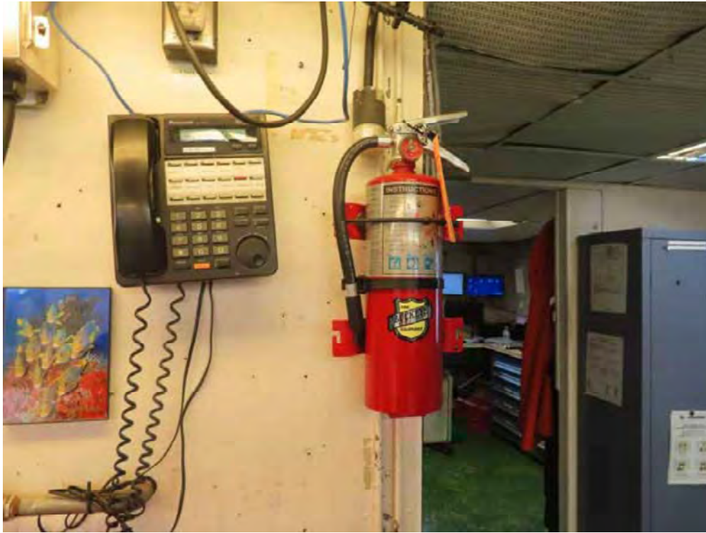
91. Typical portable fire extinguisher station
