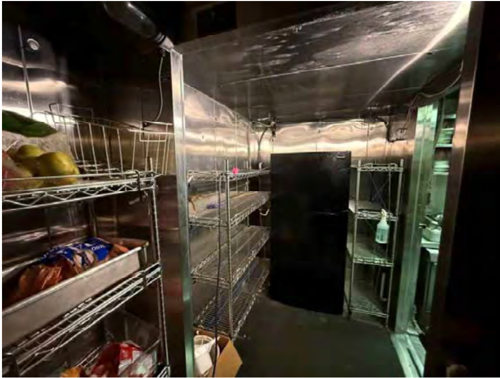
61. Deep freezer (inoperative with door removed)
