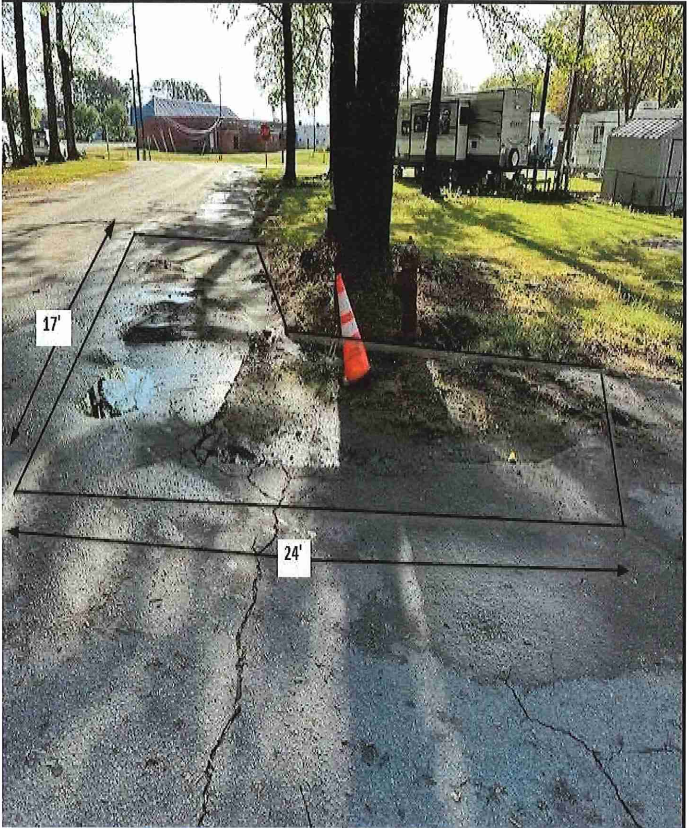
Figure 36: Perkins and Ives / Area J / This area shall be cut square before repairing the utility cut. Measurements are approximate.
