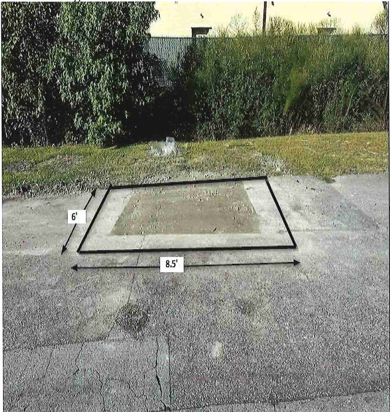
Figure 25: 219 Devonshire / Area D / This area shall be cut square before repairing the utility cut. Measurements are approximate.
