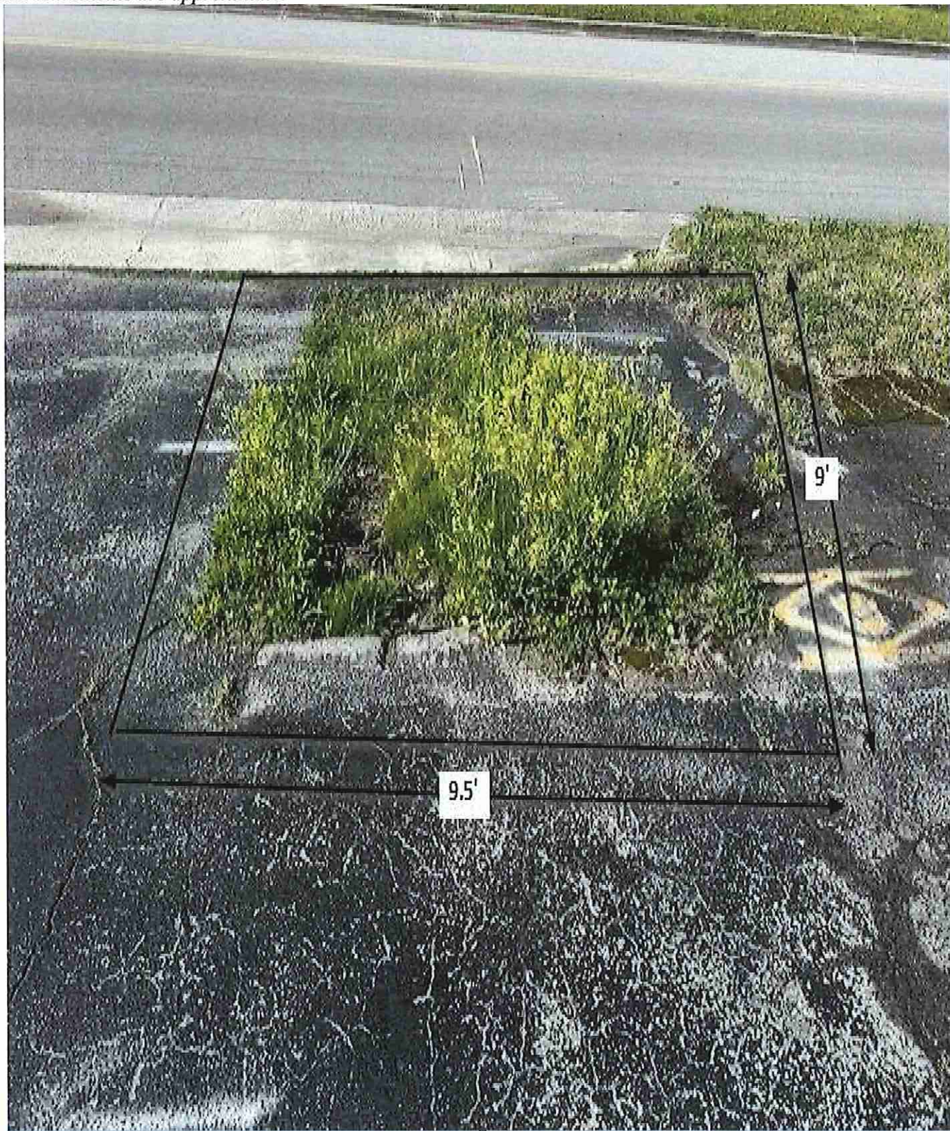
Figure 29: 112 W. Main St. / Area F / This area shall be cut square before repairing the utility cut. Measurements are approximate.
