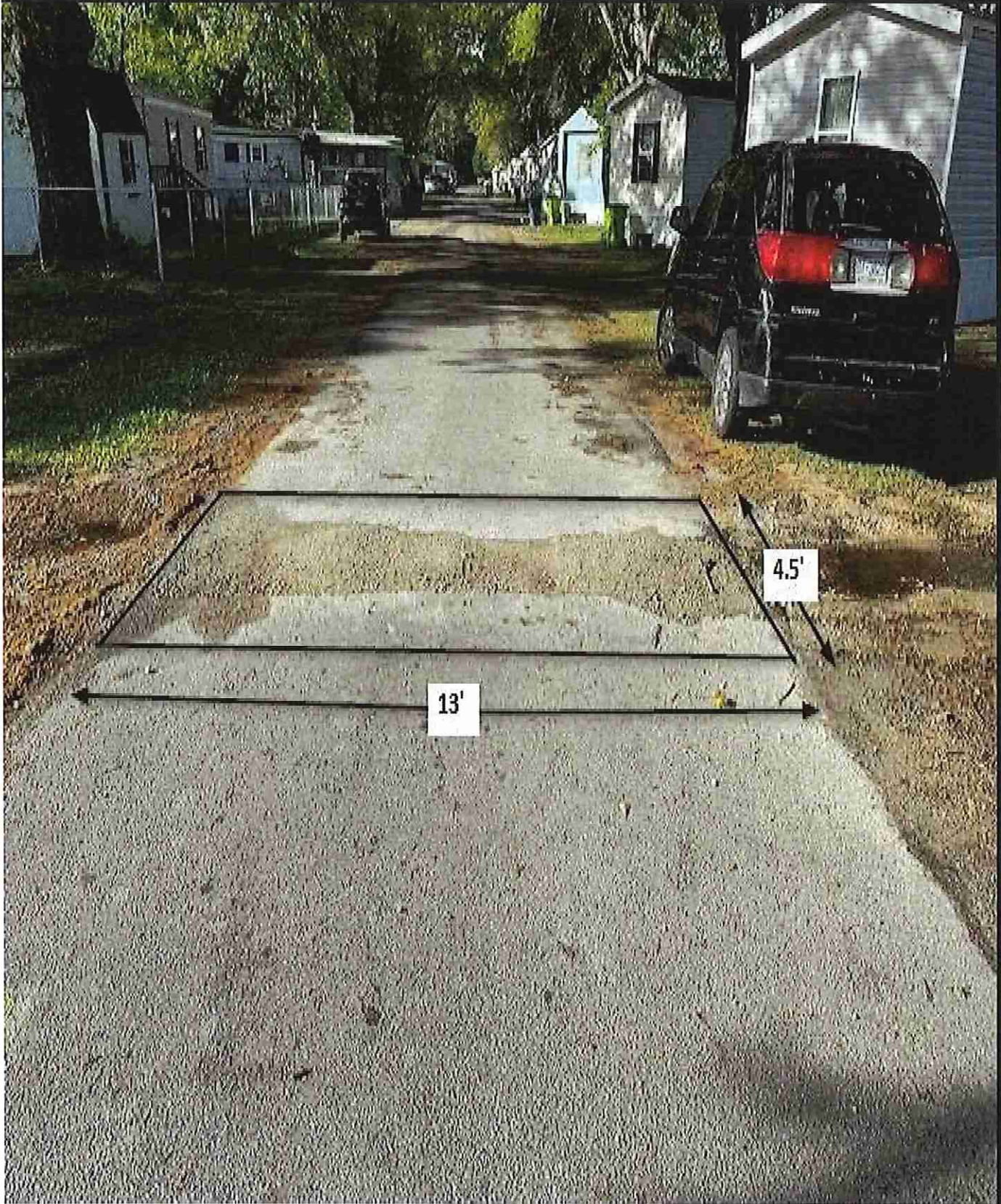
Figure 34: 208 Chestnut / Area J / This area shall be cut square before repairing the utility cut. Measurements are approximate.
