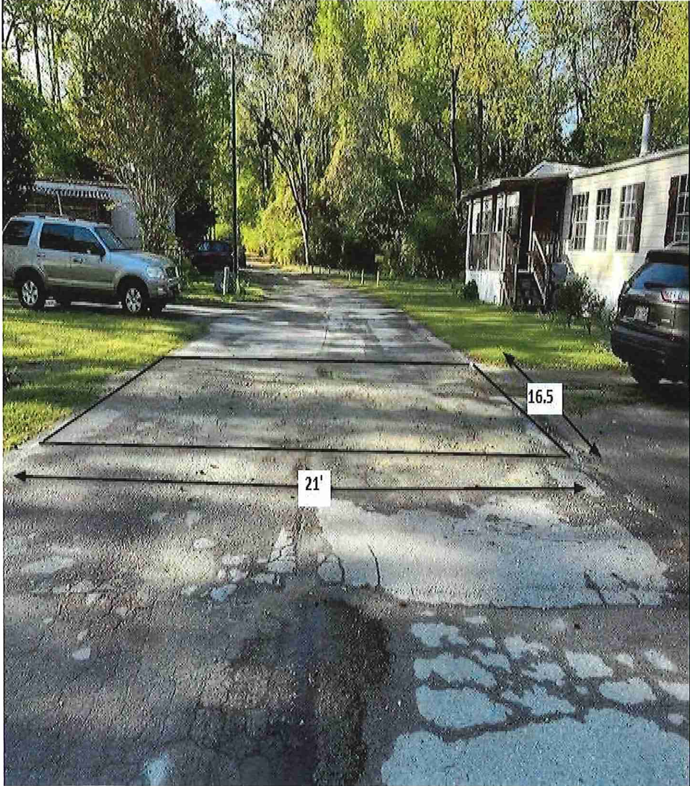
Figure 35: 228 Russel / Area J / This area shall be cut square before repairing the utility cut. Measurements are approximate.
