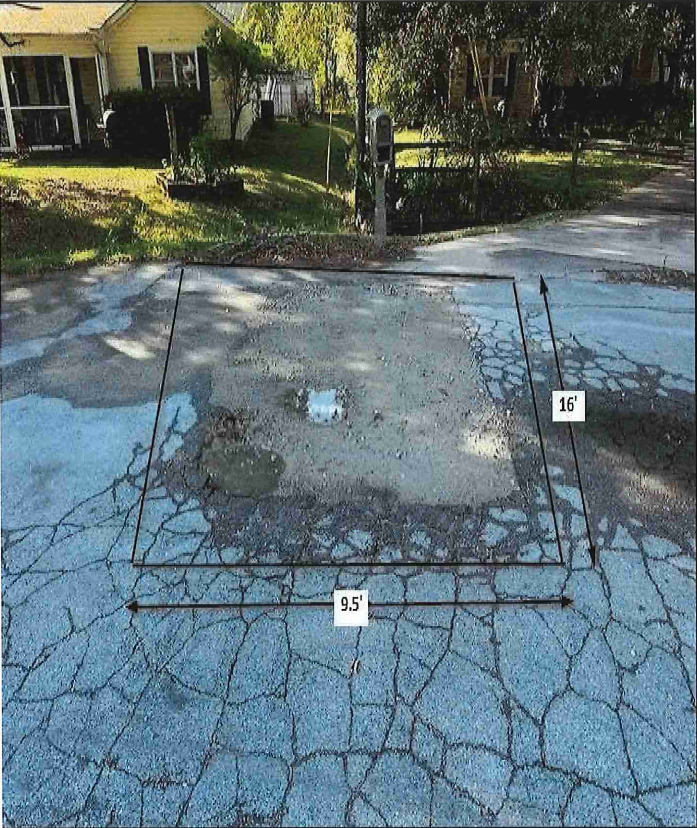
Figure 22: 109 Friar Ct. / Area D / This area shall be cut square before repairing the utility cut. Measurements are approximate.
