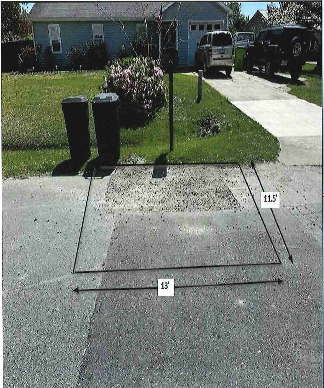
Figure 7: 104 Cindy / Area A / This area shall be cut square before repairing the utility cut. Measurements are approximate.
