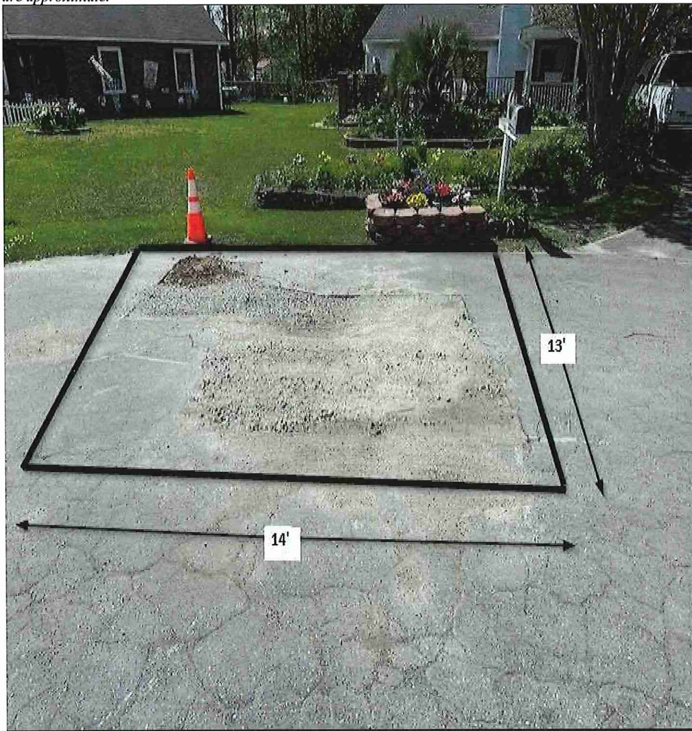
Figure 17: 522 Gene / Area A / This area shall be cut square before repairing the utility cut. Measurements are approximate.
