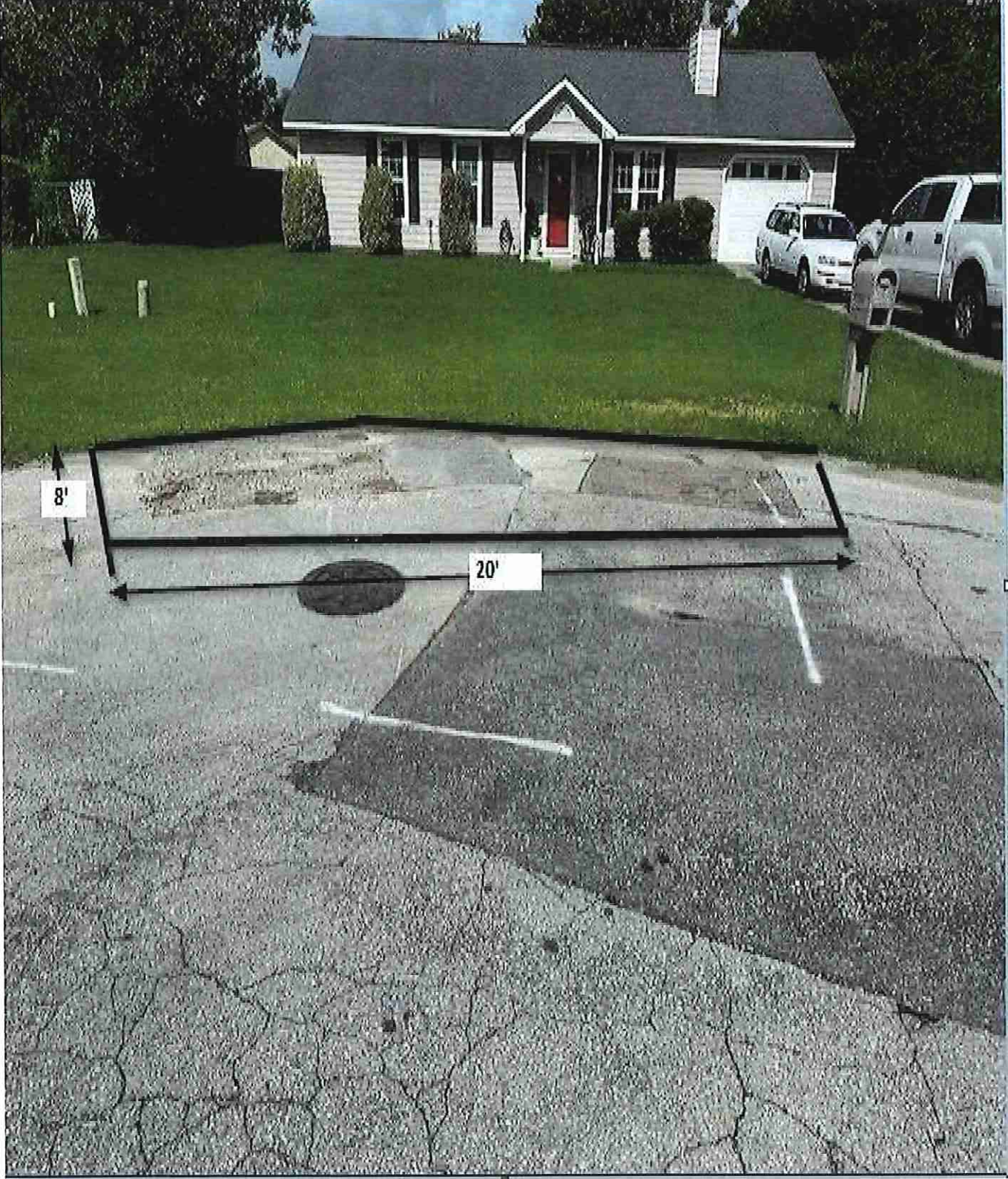
Figure 14: 401 Cottonwood / Area A / This area shall be cut square before repairing the utility cut. Measurements are approximate.
