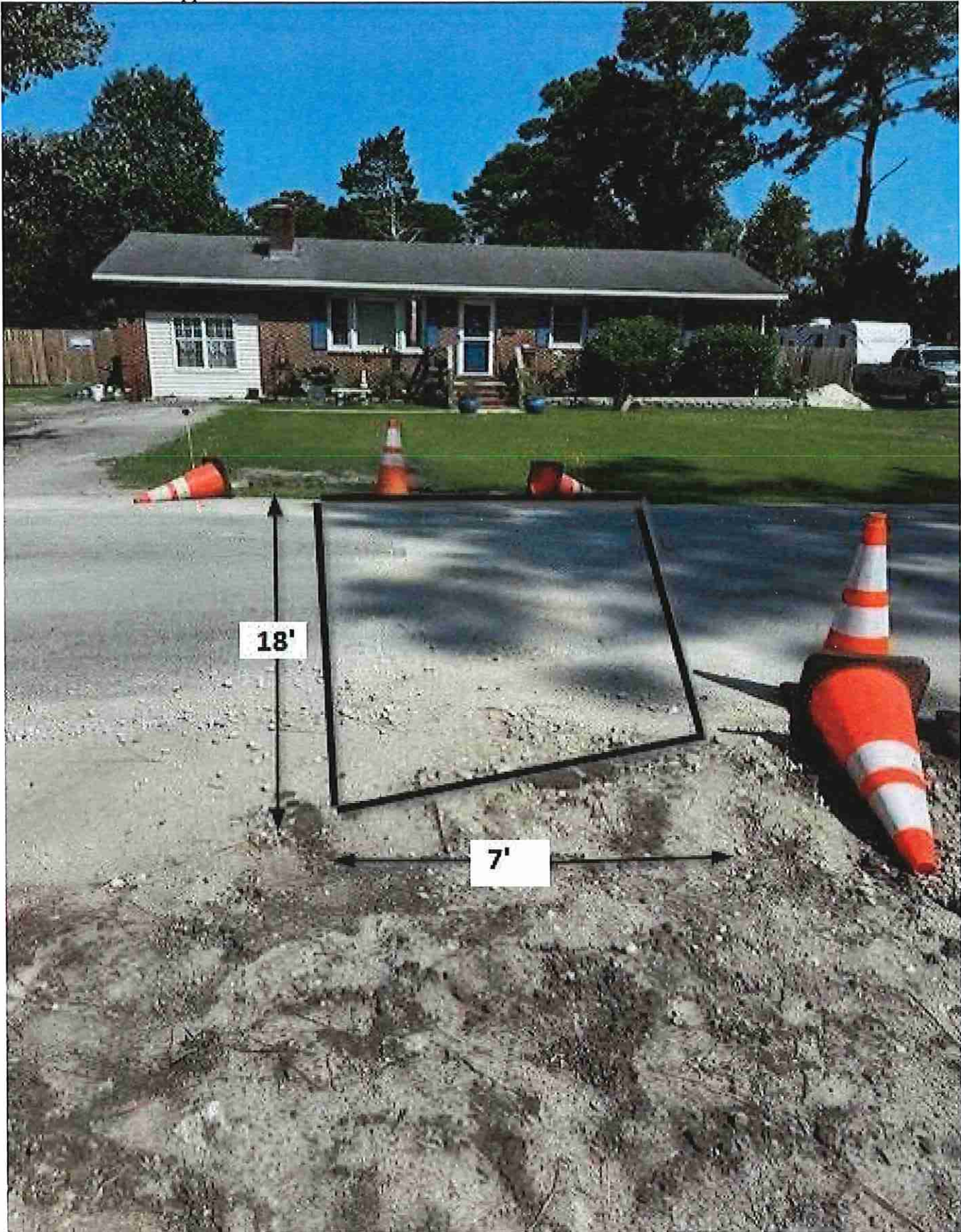
Figure 12: 205 Forest Hill / Area A / This area shall be cut square before repairing the utility cut. Measurements are approximate.
